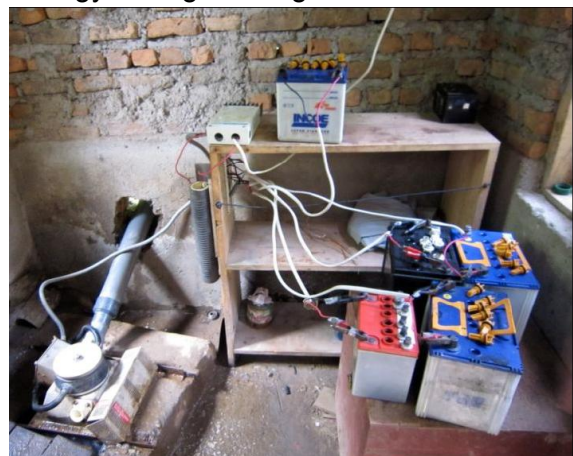
Battery charging station
