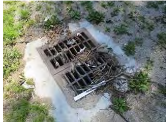
Clogged Sewer Inlet At 3011 Swope Parkway
