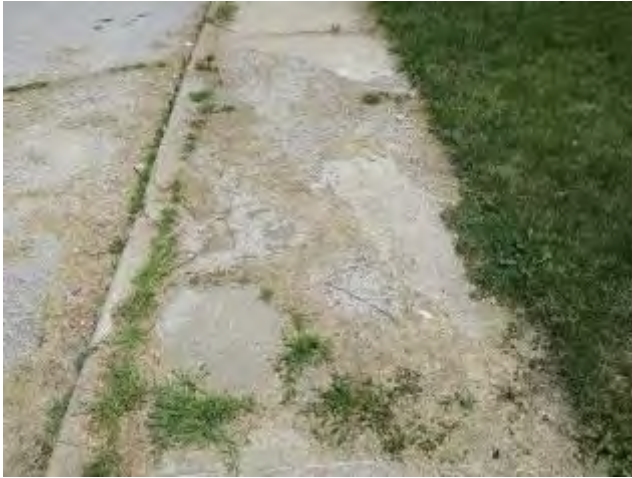
Deteriorating Sidewalk At 2801 Swope Parkway
