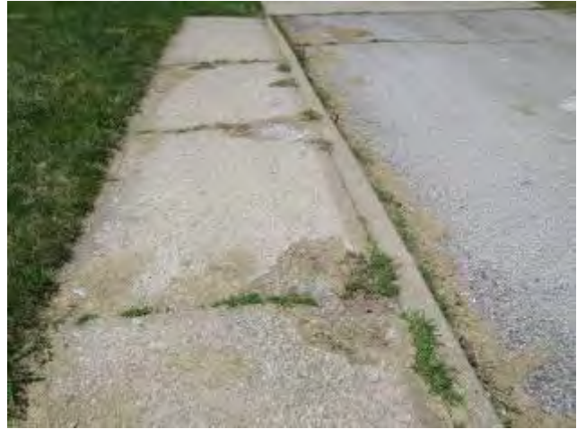
Deteriorating Sidewalk At 2801 Swope Parkway
