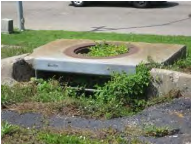
Clogged Sewer Inlet At 3011 Swope Parkway
