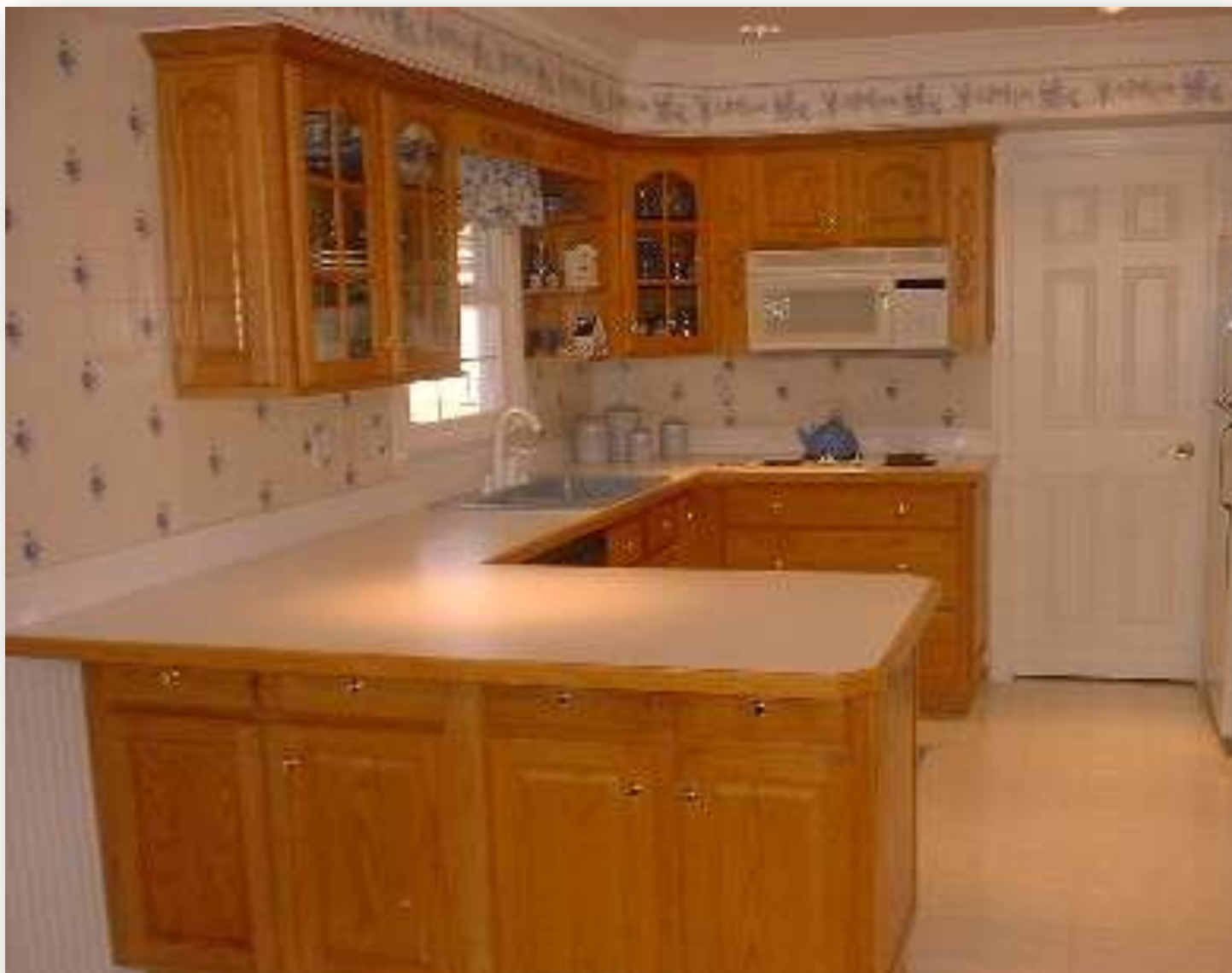
Damaged cabinets and countertop
