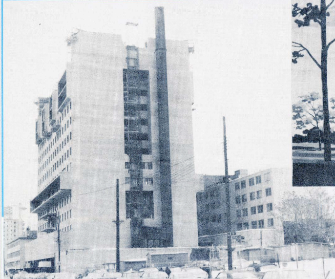
Brookdale Hospital, Flatbush, Brooklyn
