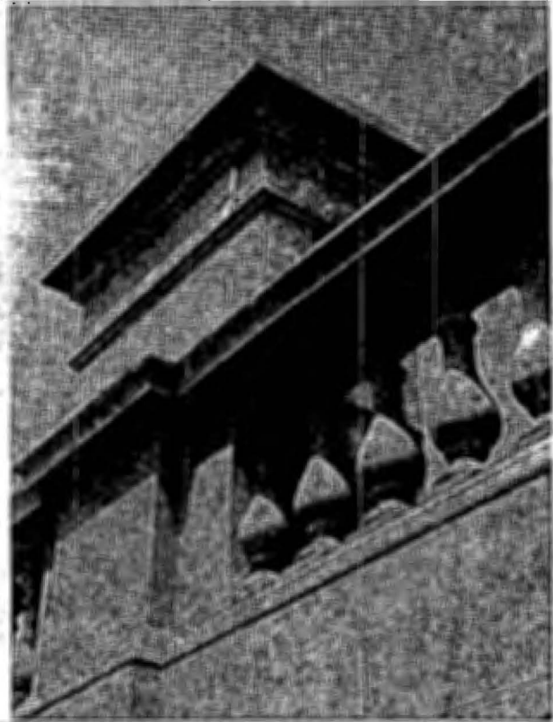
Fig. 23 Typical carved stone balustrade of the White House. Many of the original sandstone balusters have been replaced over the years (mainly with Indiana limestone), as their extreme exposure makes them susceptible to damage. photo: Tim Buehner, NPS.
