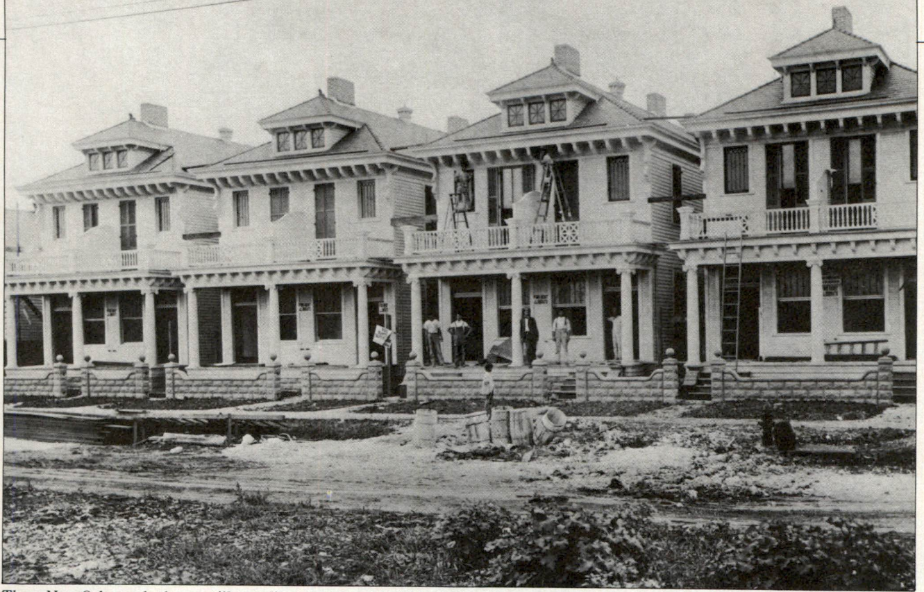
These New Orleans duplexes, still standing today, were built to fulfill Arthur P. Boh's first contract in 1909. With his brother Henry he went on to build a $150 million business.
