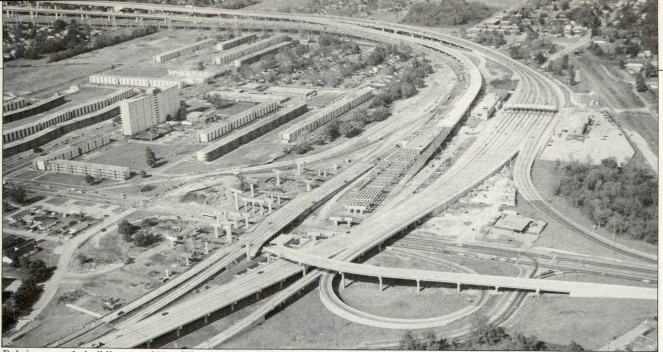
Boh is currently building two $35 million projects on the west bank of the Mississippi River. Shown here is the West Bank Approach to Greater New Orleans Mississippi River Bridge No. 2.
