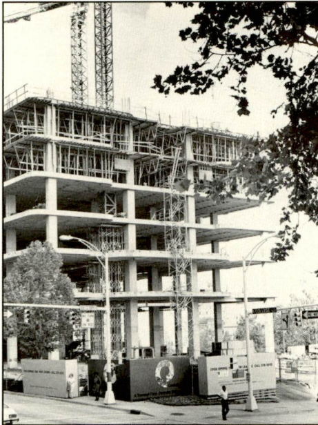
More than $7 billion in new construction has taken place in Charlotte since 1981.
