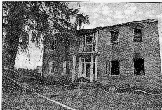
The 173-year-old house, which is listed on the National Register of Historic Places, might have to be torn down because of the damage, said Georgetown Fire Chief Terry Herthel.
