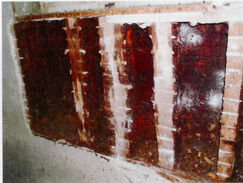
Detail of interior framing and cladding under brick veneer. Image from upper-half story of wing block.
