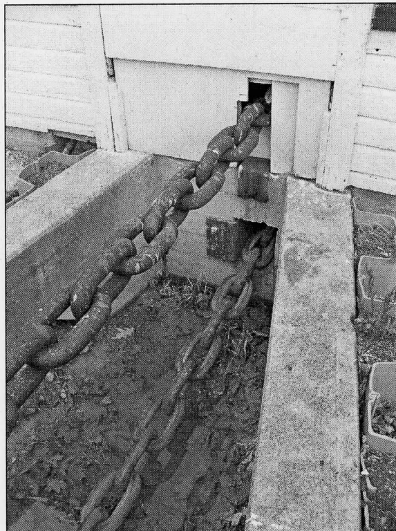
Illustration 10: Five-foot-deep, Y-shaped foundation below grade at south elevation of head house, showing in-haul chain as it leads to front of cradle
