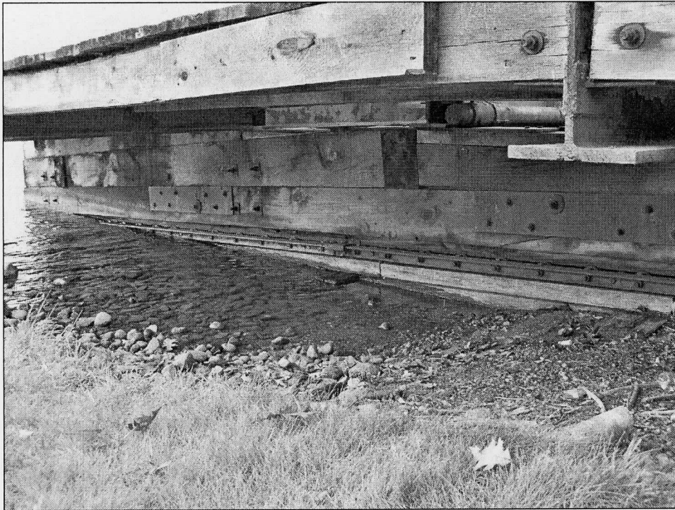
Illustration 11: Underside of the partially submerged cradle showing the roller racks and the foundation supporting the track plates upon which the roller frames sit
