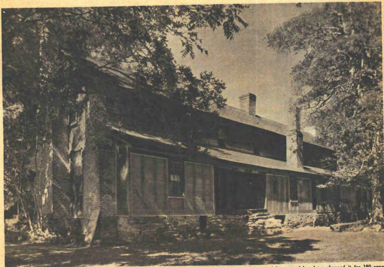
Where weatherboards have been removed, a temporary covering of polyethylene shows how the house grew and how remodelers have changed it for 180 years.
