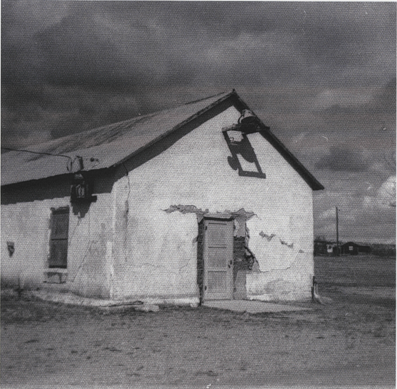
Figure 13. Photograph of the Arivaca Schoolhouse in 1973, view to the northeast (courtesy Mary Kasulaitis, Arivaca).
