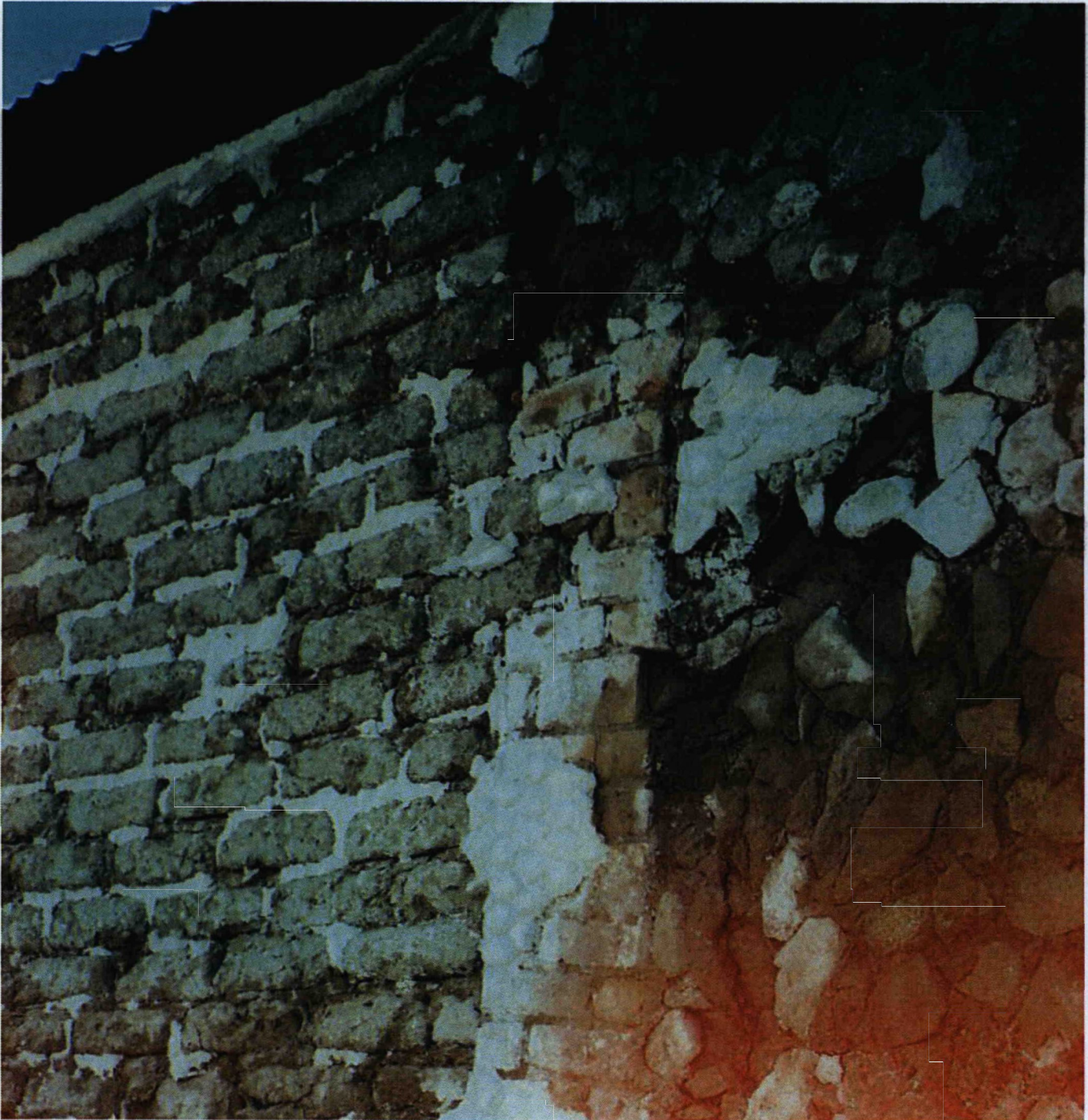
Figure 7. View of the joint exposed along the exterior west wall of the schoolhouse during the 1994 rehabilitation work (courtesy Mary Kasulaitis, Arivaca).
