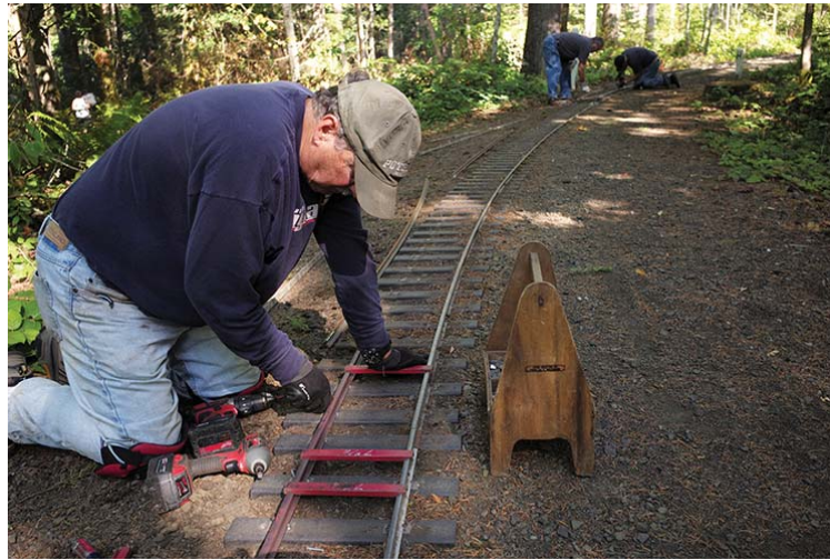
Dan Simmons is replacing worn out aluminum rail with new steel rail in the northwest park of the KLS railroad. Tom Huffman and Don Rogers are in the background.
