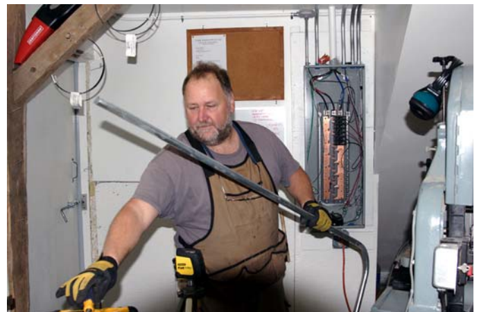
John Small working on electrical wiring in the new Workshop. Image by Al T.
