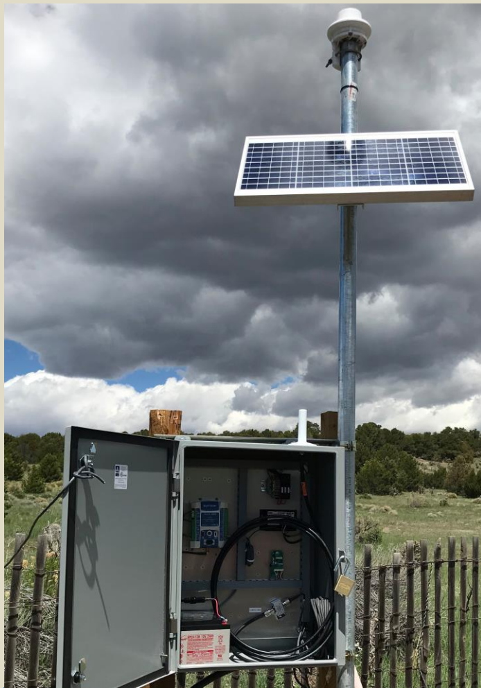
Each station includes a radar stage sensor, water surface velocity radar, disdrometer precipitation sensor, satellite data transmitter and a solar charging system.
