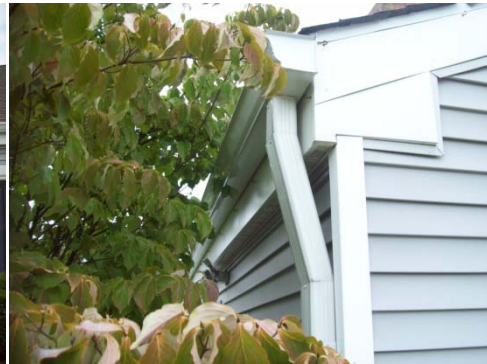
Tree growing into building
