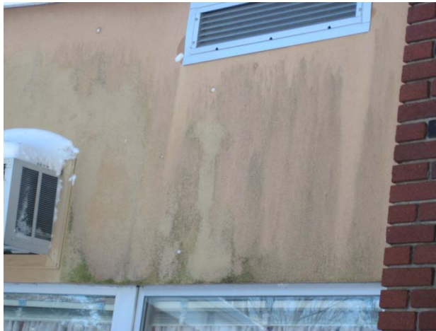
Water damage EIFS
