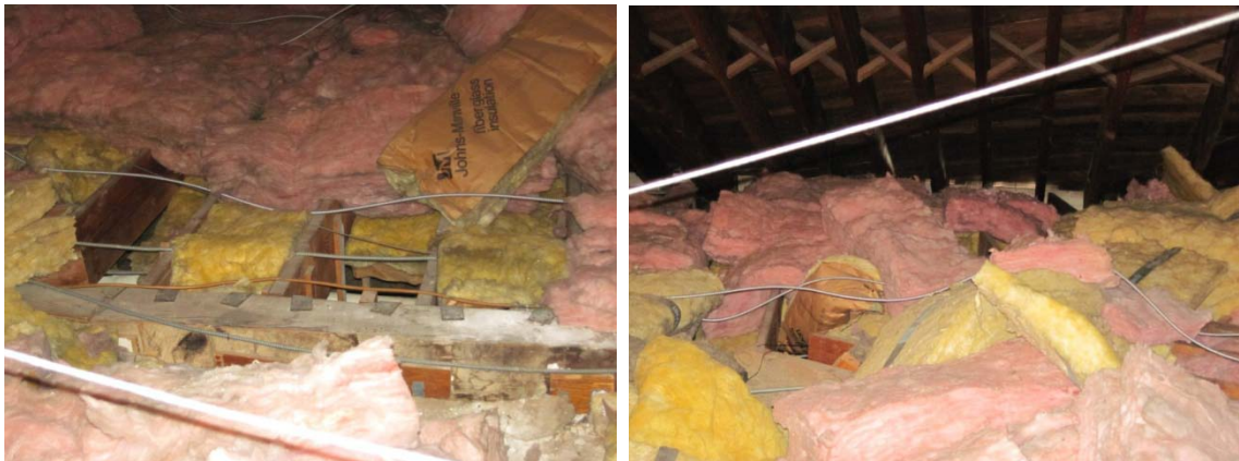
Fiberglass insulation haphazardly displaced
