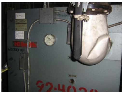
C/D wing boiler
