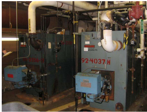
A/B wing boilers
