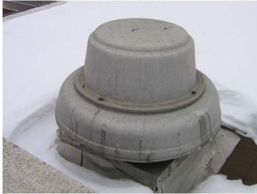
Typical Rooftop Exhaust Fan
