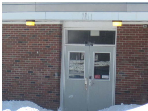
Exterior lights left on during daylight hours
