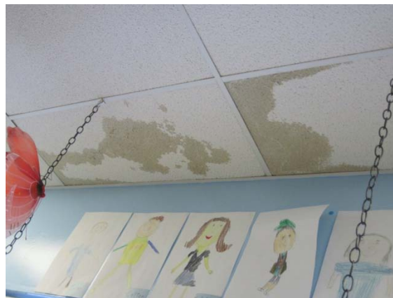
Image showing damaged ceiling tiles in classroom
