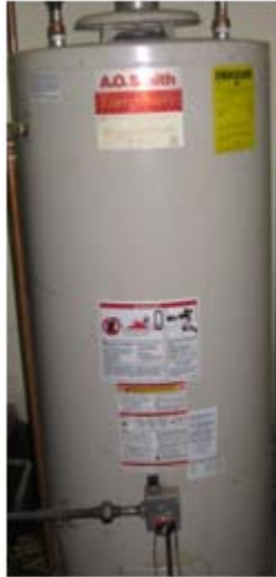
AO Smith water heater
