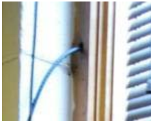
Un-caulked/un-sealed exterior wall penetrations
