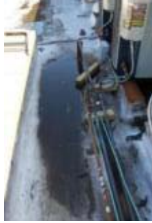
Signs of standing water/pooling
