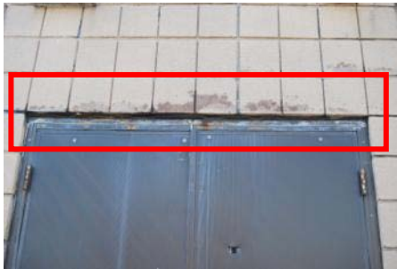
Rusted and deteriorated steel lintel with associated signs of water damage.
