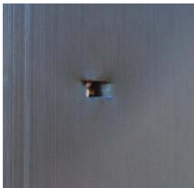
Damaged metal door panel
