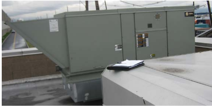
Trane gas-fired outdoor unit heater
