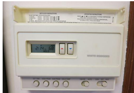
Image 8: Thermostat Control in Front Office Area
