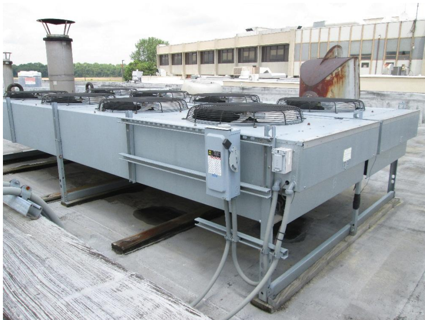
8. Air cooled condenser for space cooling
