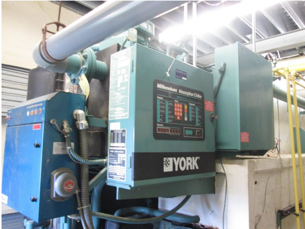
3. Existing absorption chiller
