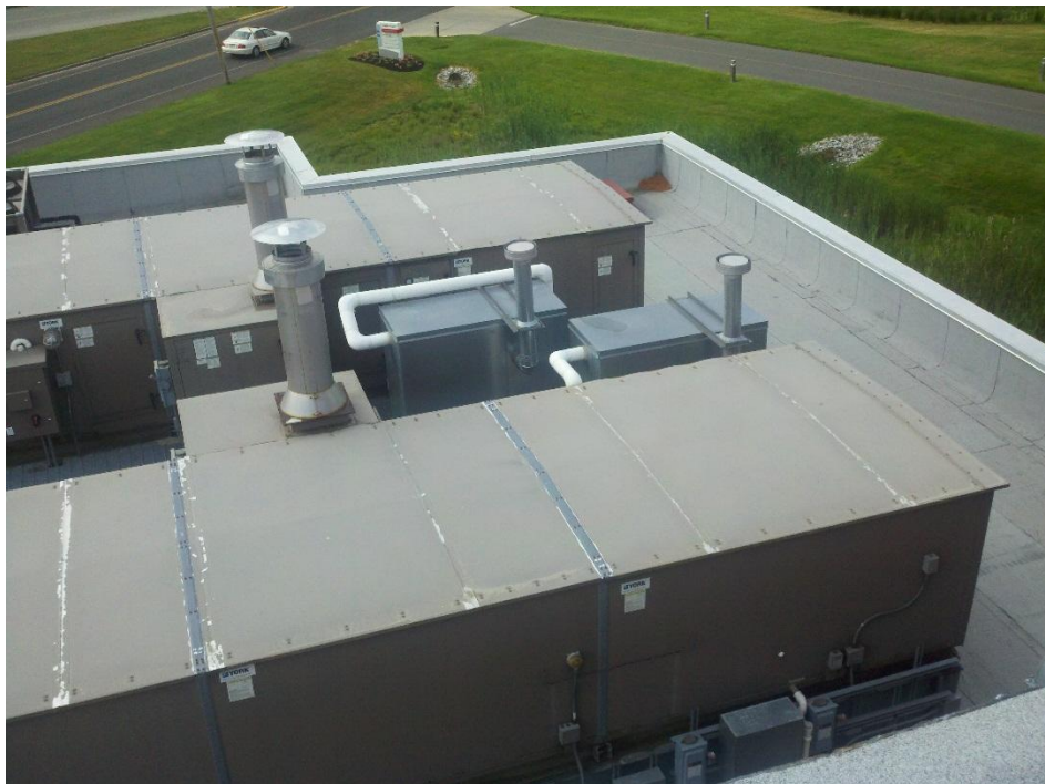
2. Existing rooftop air handling units
