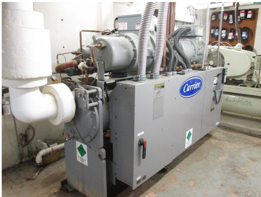
6. Existing centrifugal chiller
