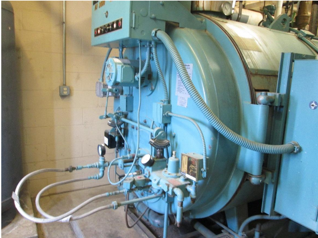
5. Steam boiler in utilities building (typical of 3)
