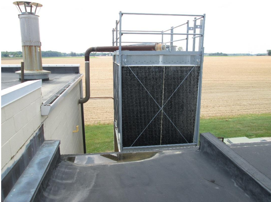
7. Cooling tower behind utilities building
