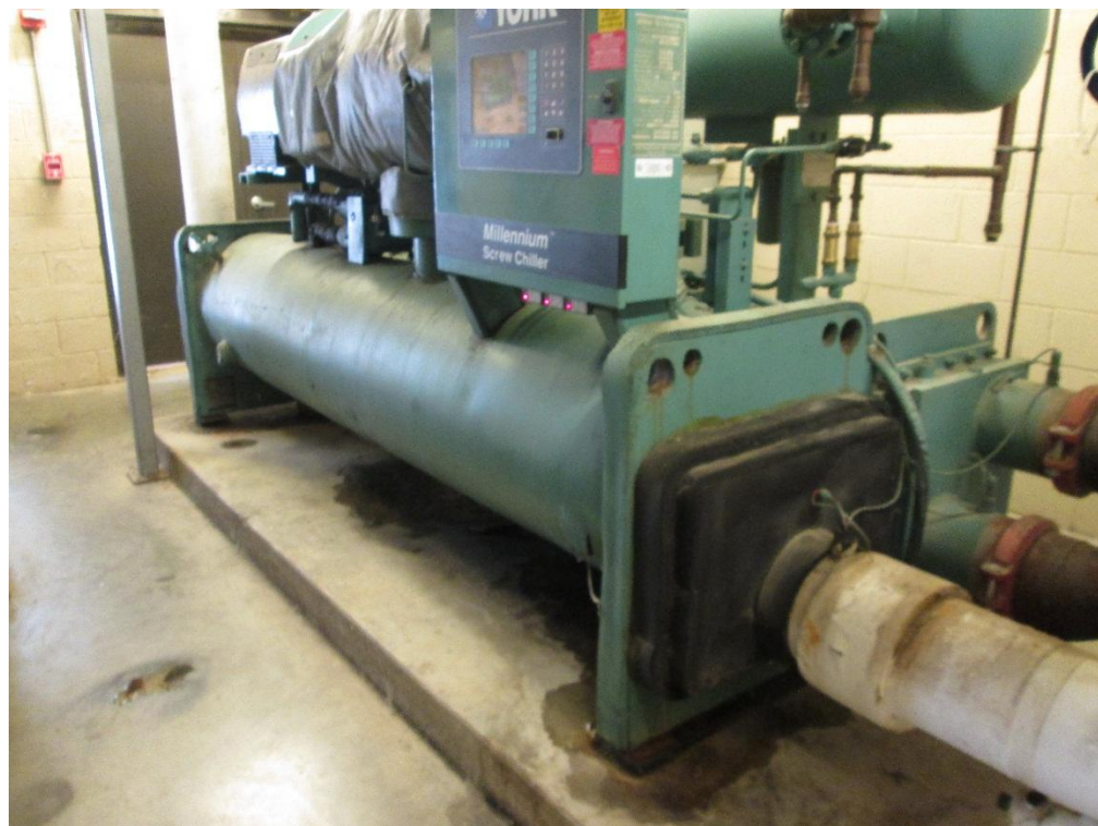
4. Existing centrifugal chiller
