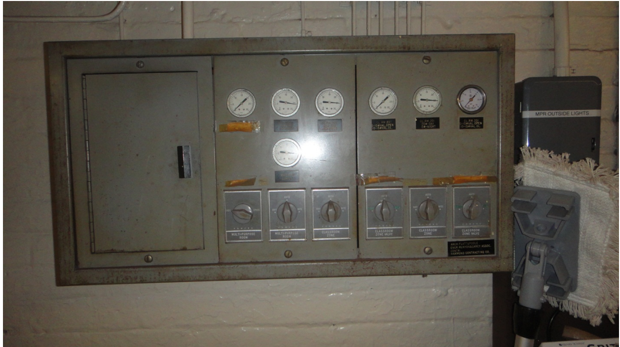
PNEUMATIC SYSTEM CONTROL PANEL
