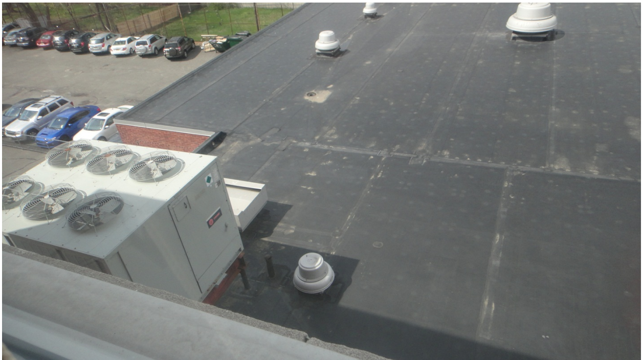
AIR COOLED CHILLER ON ROOF
