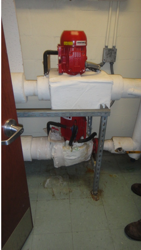
CHILLED WATER PUMPS
