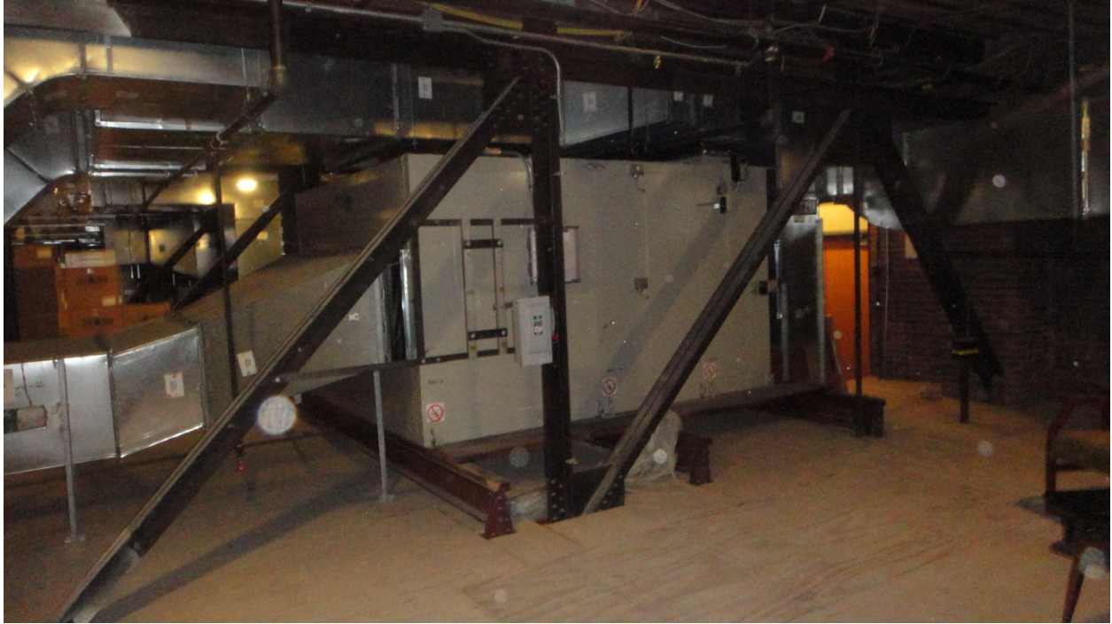
AIR HANDLING UNIT
