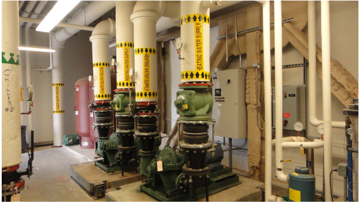
HOT WATER PUMPS
