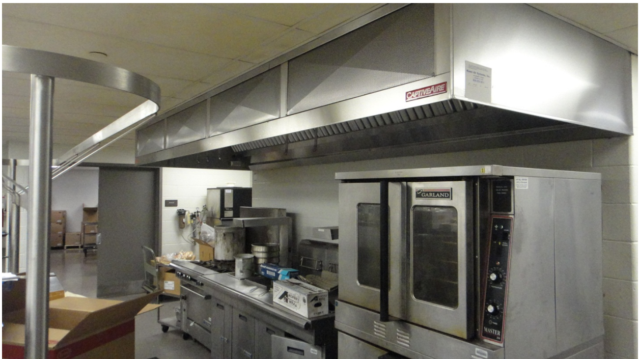
KITCHEN EXHAUST HOOD
