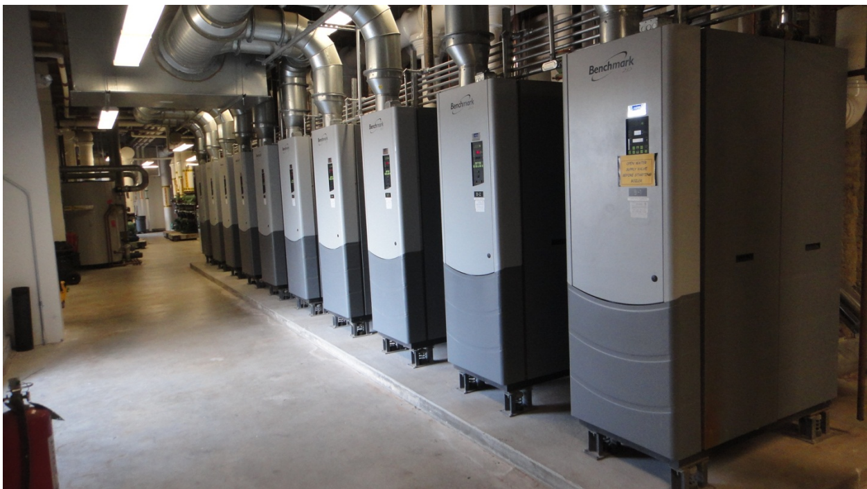
HOT WATER BOILERS
