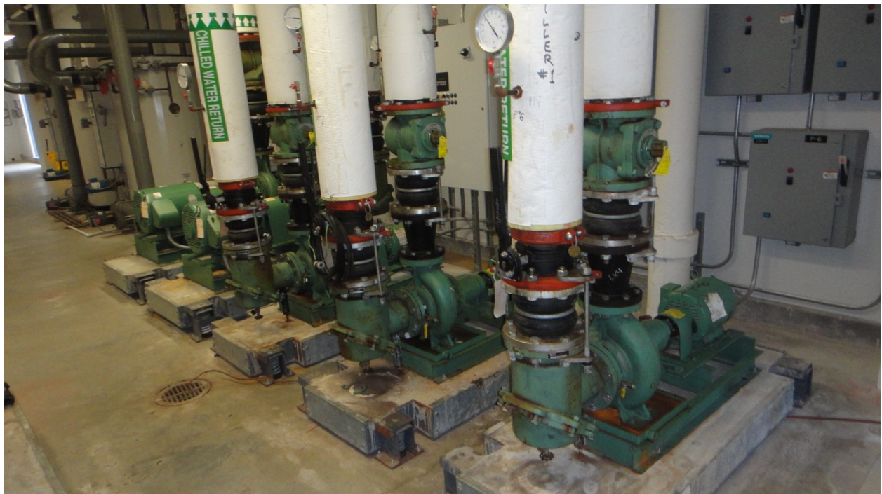
PRIMARY AND SECONDARY CHILLED WATER PUMPS
