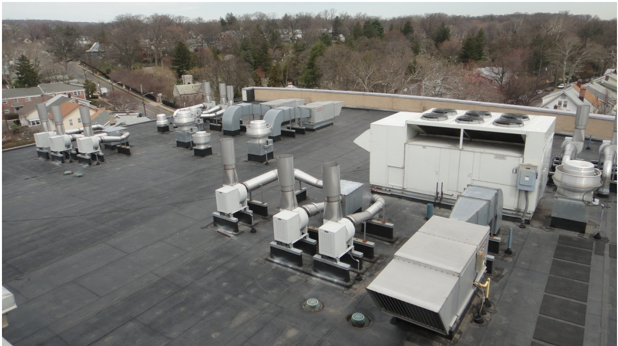
ROOFTOP UNIT, MAKE UP AIR UNITS, LAB EXHAUST FANS AND GENERAL EXHAUST FANS
