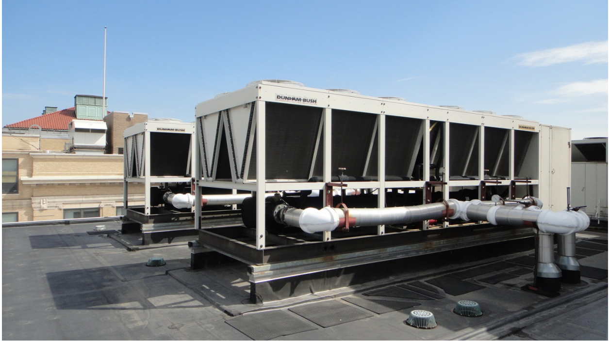
AIR COOLED CHILLERS
