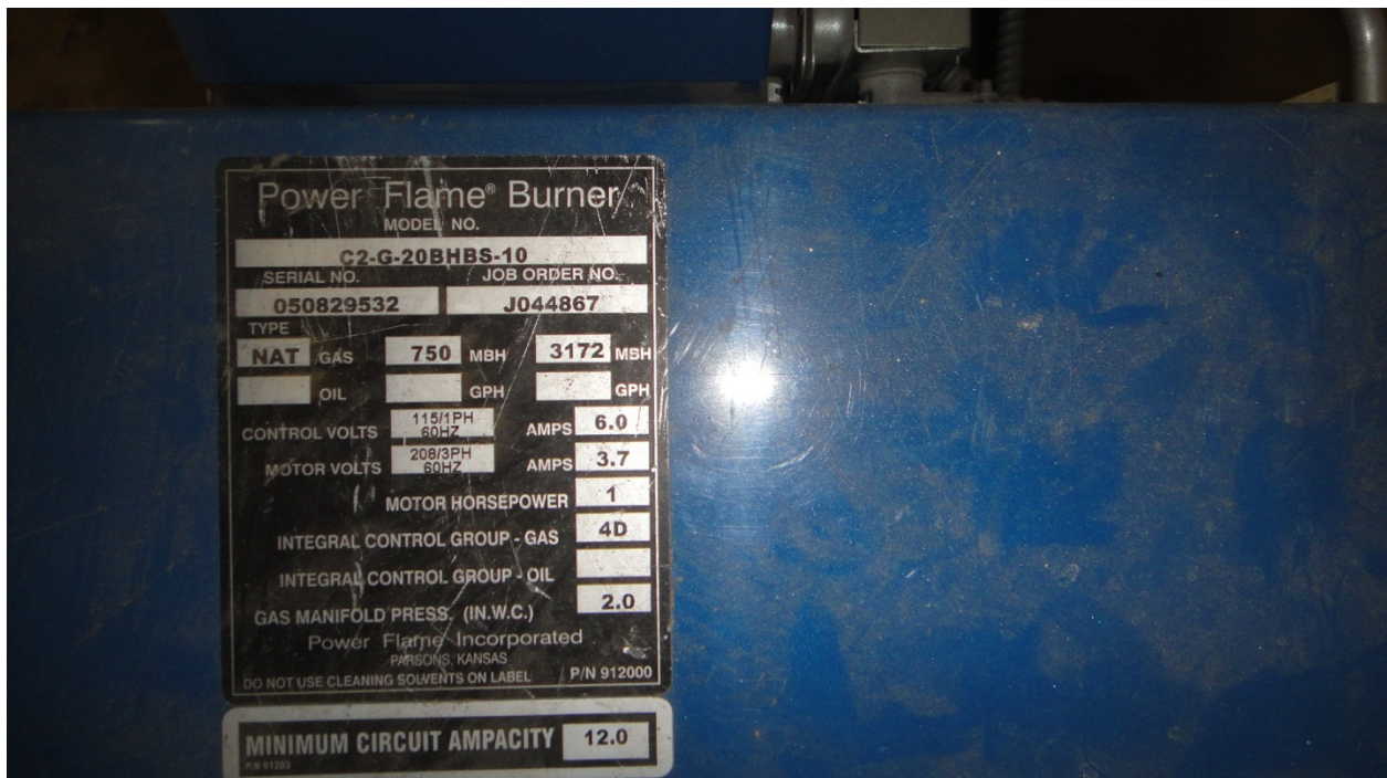
BOILER BURNER NAMEPLATE
