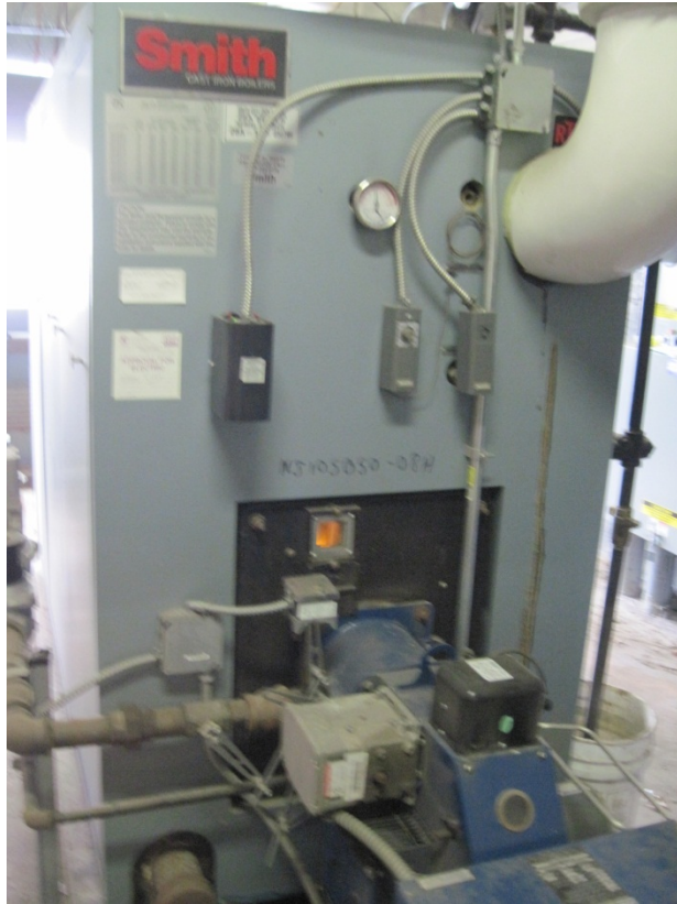
HOT WATER BOILER
