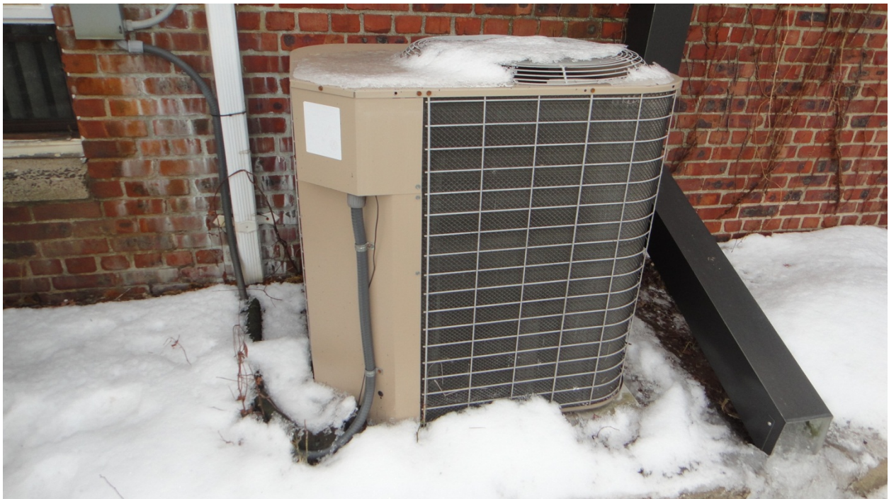
AIR COOLED CONDENSING UNIT SERVING OFFICES
