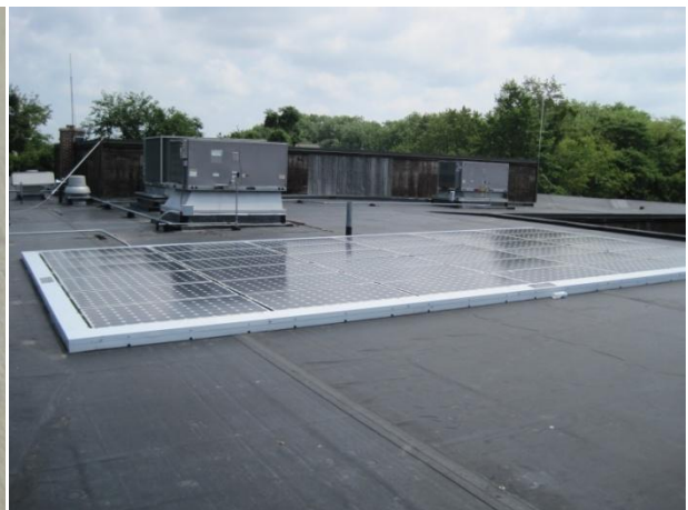
Rooftop mounted 7.5 kW PV system
