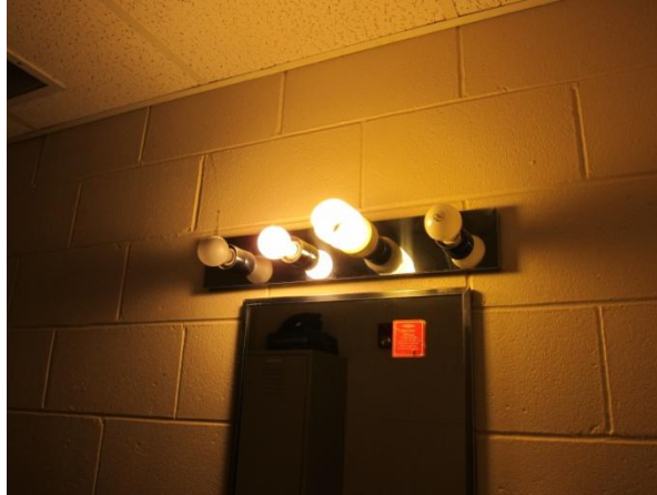
Compact Fluorescent and Incandescent bulbs on bathroom fixture
