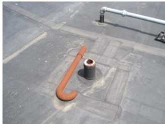
Rusted and broken exhaust pipe can damage rubber roof finish
