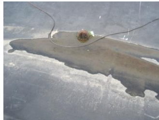
Vegetation growth on roof and puddles
