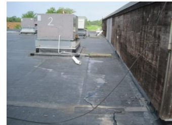
No drainage route for condensate pipe
