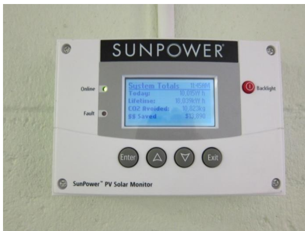
SunPower PV Solar Monitor
