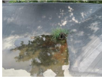
Vegetation growth on roof and standing water
