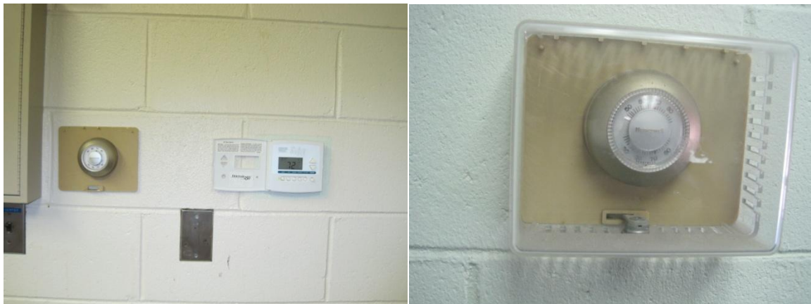
Manual and programmable in the building
