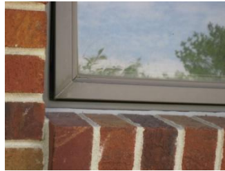
Window obstructed from totally closing
