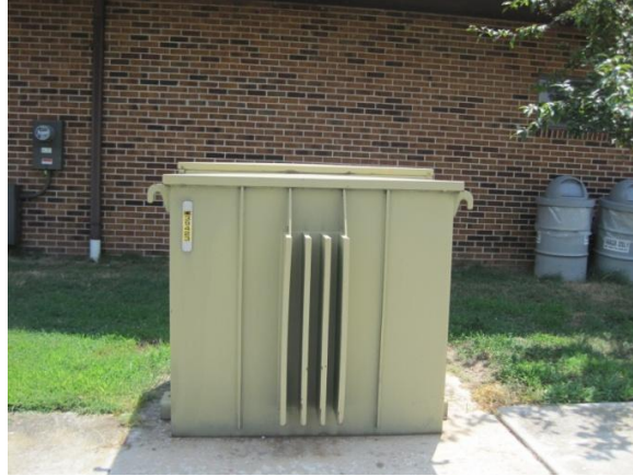
Incoming power main transformer
