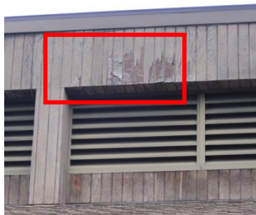
Deteriorating exterior wall finishes
