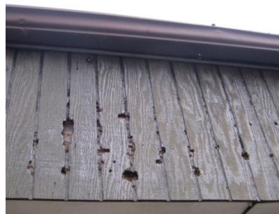
Insect damage/nesting in exterior wall finishes
