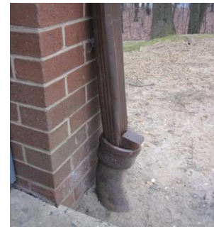
Uncontrolled roof water run-off due to temporary/open downspout drain connection
