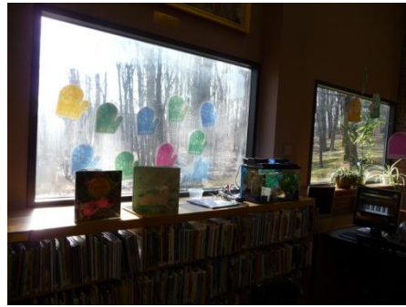
Main Library area window fogged with moisture trapped between the panes
