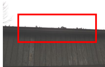
Clogged gutters and downspouts
