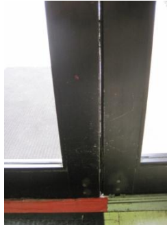
Missing/worn weather stripping
