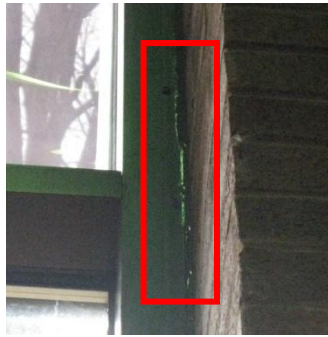
In the lower floor area an ineffective insulation and caulk window to wall connection detail was detected, showing daylight
