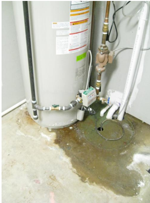
Leaking DHW heater
