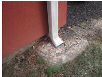
Uncontrolled roof water run-off due to missing/ ineffective downspout deflector
