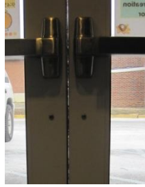
Missing/ worn weather stripping
