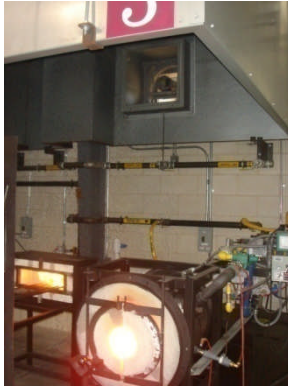
Picture: Showing Landfill Gas Piping
