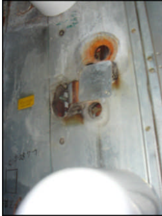
Picture: Davidow AHU -1
