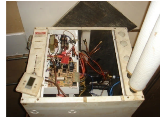
Picture: Tillis Hall Heat Pump
