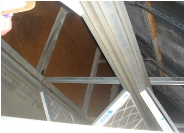
Picture: Davidow Hall - AHU – 4
