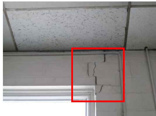
Cracks between cement blocks on interior wall indicating potential structural damage
