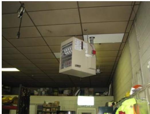
Typical Natural Gas Unit Heater with flue piped to roof
