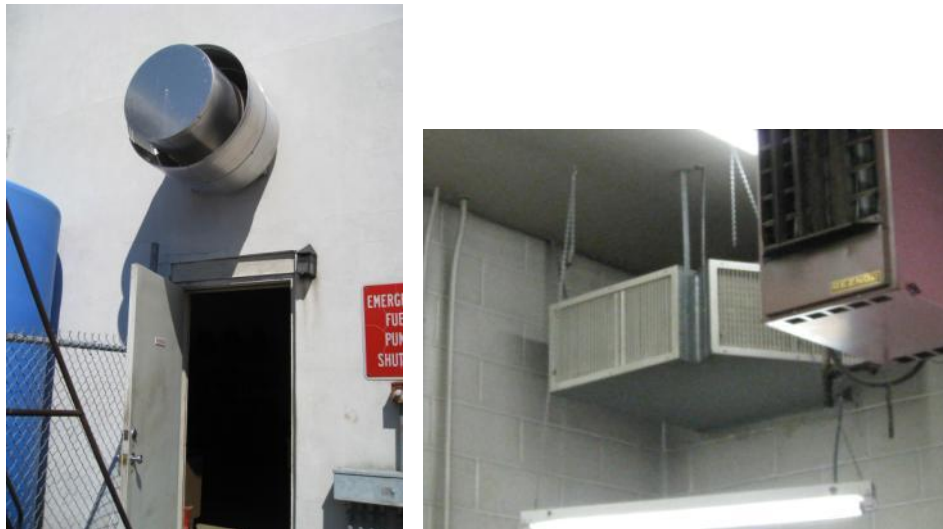
Outside Air Ventilation System exhaust fan (left); Outside air supply ducts (right)
