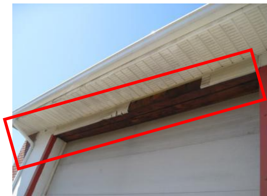
Missing/deteriorating siding on garage door header
