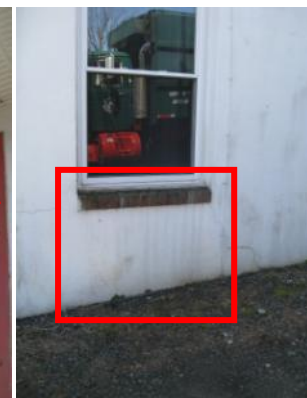
Cracked stucco showing signs of water or moisture damage
