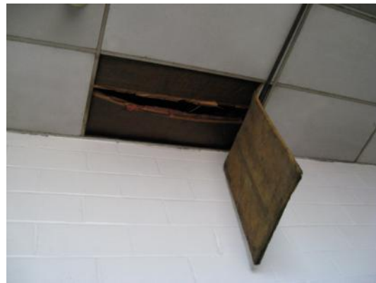
Sagging/damaged ceiling tiles in many areas
