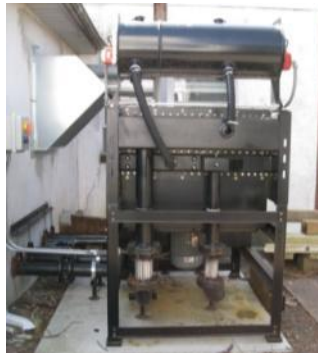
GE cooling system for generator
