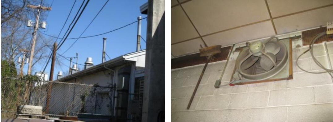
Rooftop Exhaust fans visible from outside (left); Typical through the wall garage exhaust fan (right)
