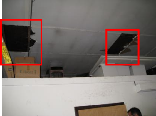
Missing gypsum wallboard visible in the interior
