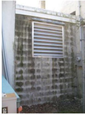
Damaged exterior wall finishes
