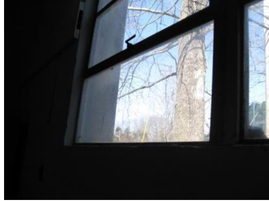
Single-glazed window with ineffective frame
