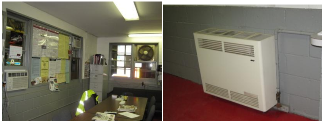
Break Room AC units and exhaust fan (left), Furnace (right)
