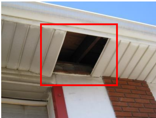
Missing panels on eave
