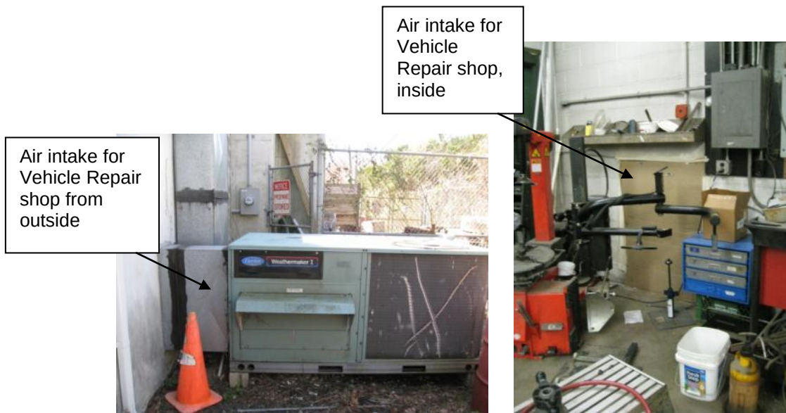
Vehicle Repair Garage RTU for cooling (left) and boarded up air intake (right)
