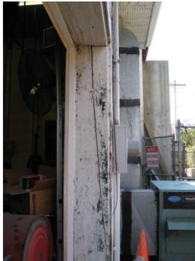
Damaged/aged door frame on rear truck garage door
