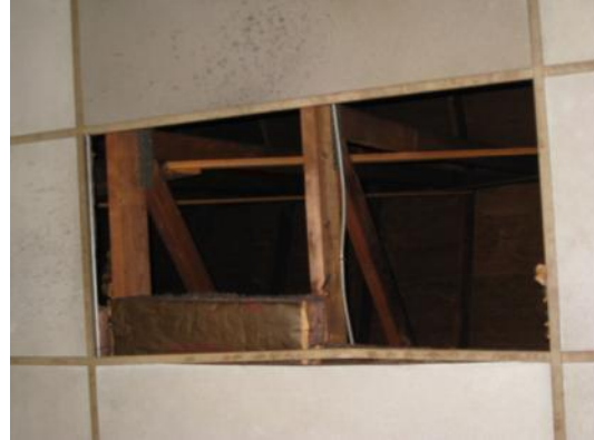
Uninsulated attic above drop ceiling open to occupied space due to missing gypsum wallboard and damaged ceiling tiles
