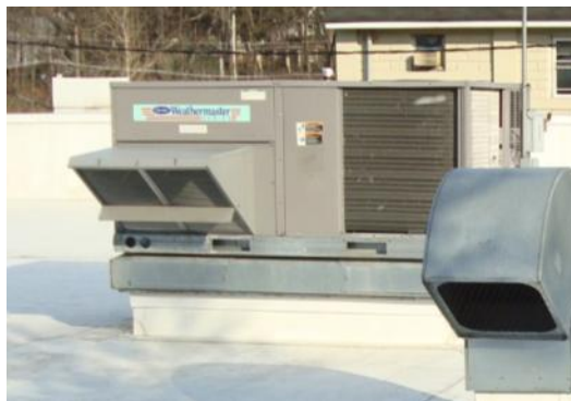
Carrier Weathermaster Rooftop Unit
