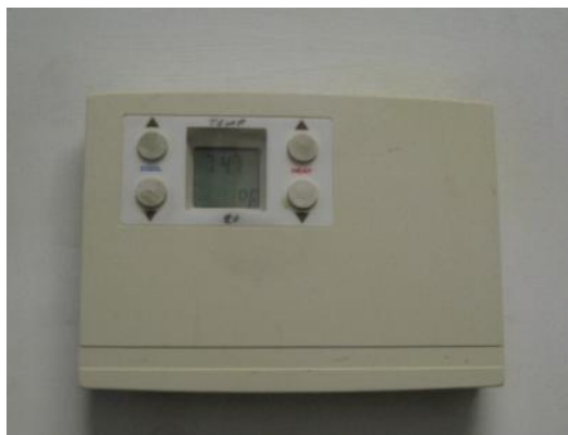
One of many temperature sensors
