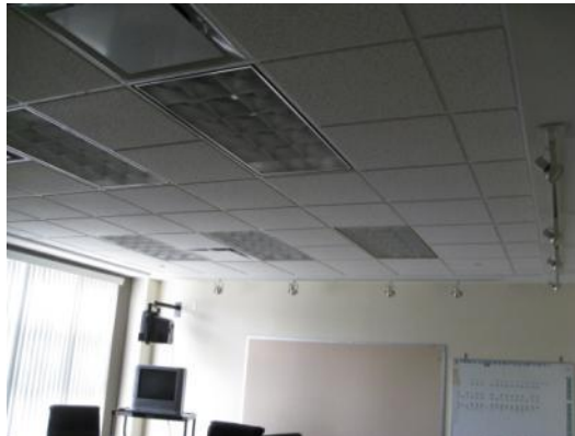
T8 Fixtures and Halogen Track Lights
