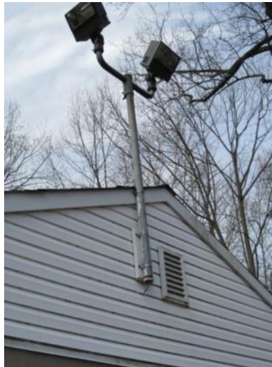
Metal Halide Fixture mounted on exterior wall
