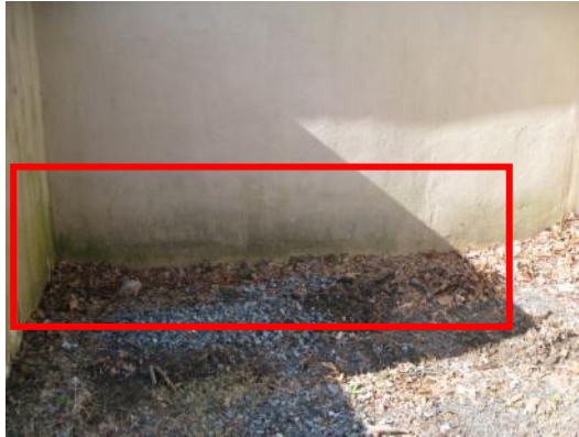
Moisture damage at base of exterior wall
