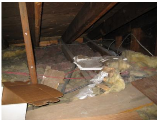
Uneven attic insulation found
