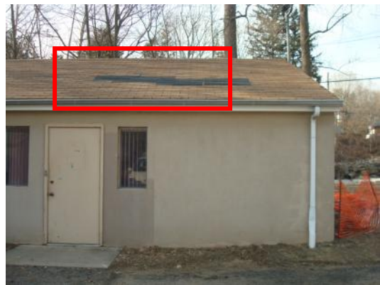
Missing/damaged roof shingles
