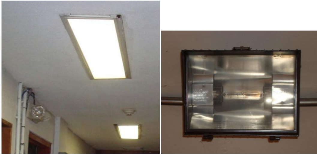
Space lighting, T12 fixtures (left); Shooting range Metal halide fixtures (right)
