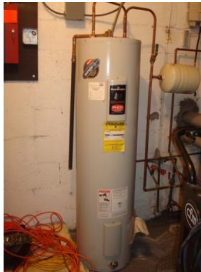
DHW Heater in Mech Closet
