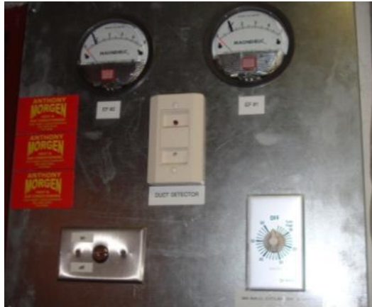
Exhaust System Control Panel
