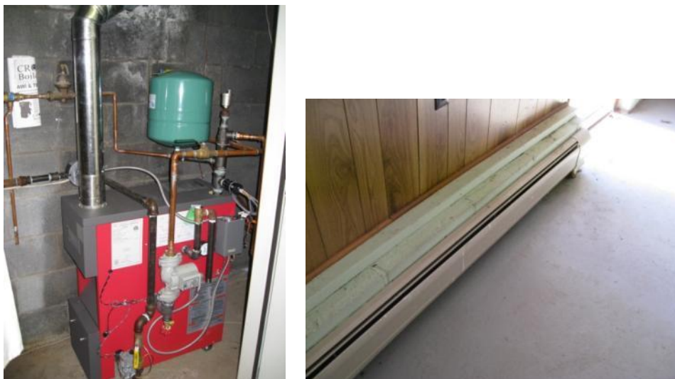
Crown Hot Water Boiler and Perimeter Baseboards
