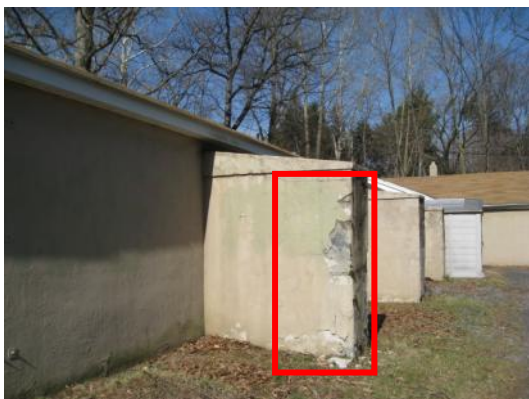
Damaged stucco finish
