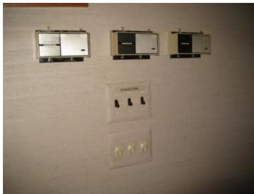
Three thermostat controls (top), three exhaust fan switches (middle) and speed control for each exhaust fan (bottom)
