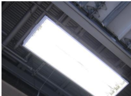
Ceiling suspended T5 fixtures in garage
