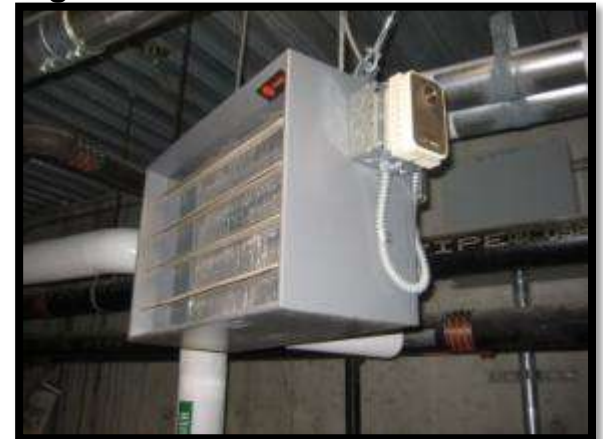
Unit Heater at Charles Smith that cycles on excessively
