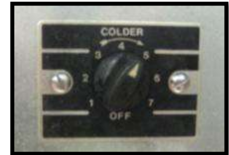
Kitchen cooling counter left on during building unoccupied hours
