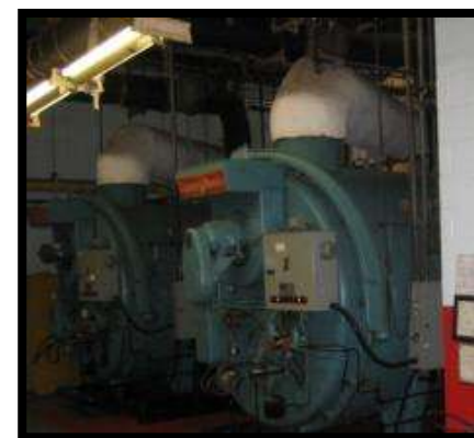
High School Steam Boilers
