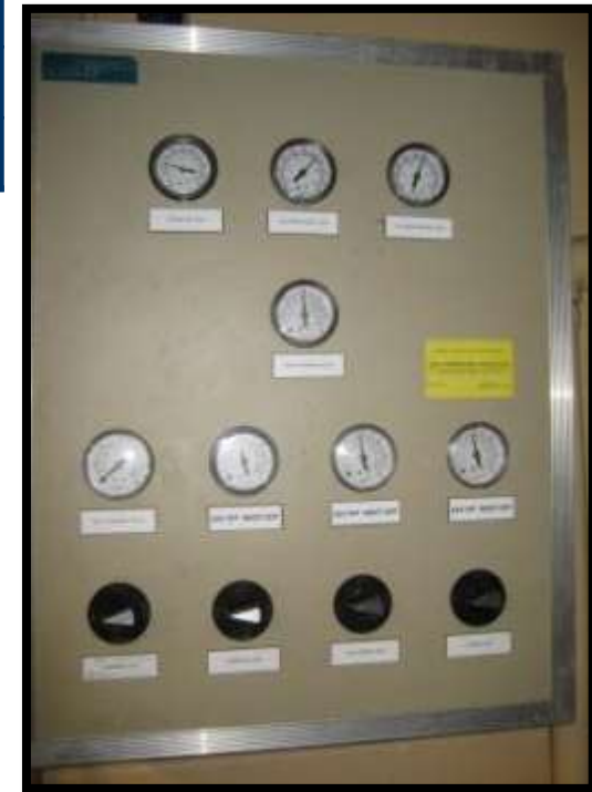
Pneumatic control panel at Lindbergh Elementary
