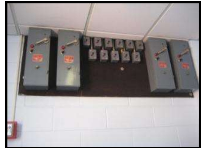
Exhaust fan manual switches left on 24/7
