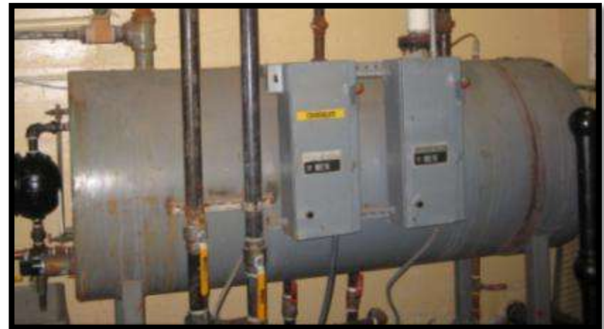
Uninsulated condensate return tank in Lindbergh Elementary School
