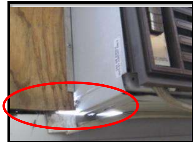
Window AC with outside air leakage in the library at the High School
