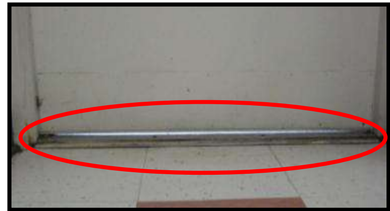
Close up of an exterior door with no weather stripping in a science room at Lindbergh Elementary School
