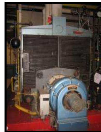
Lindbergh Steam Boiler
