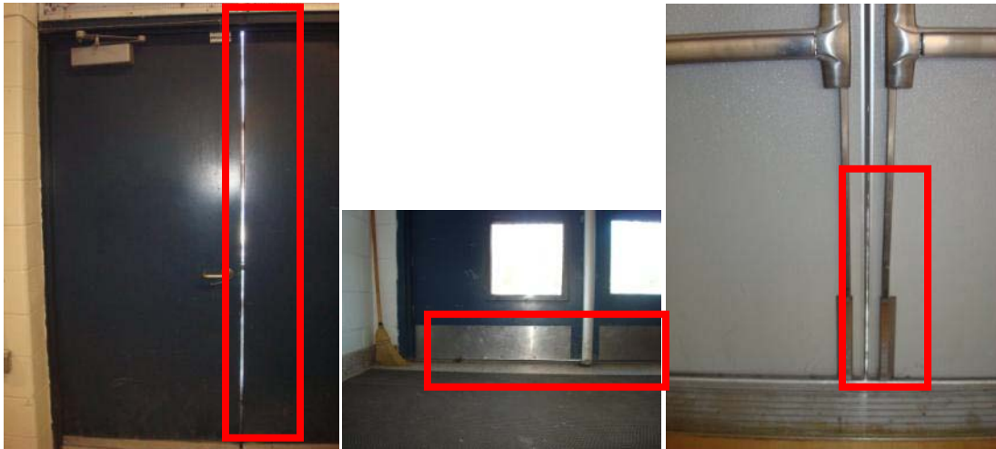
Various exterior door areas needing weather stripping
