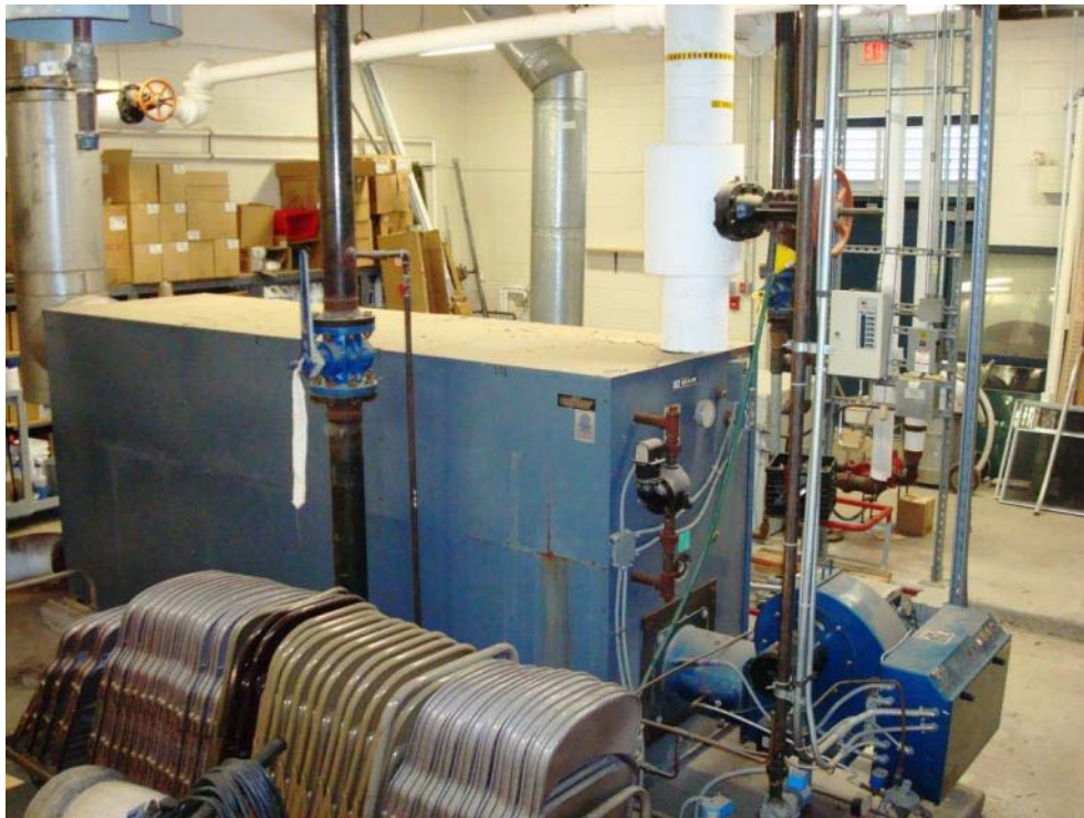
Weil McLain Natural Gas Boiler
