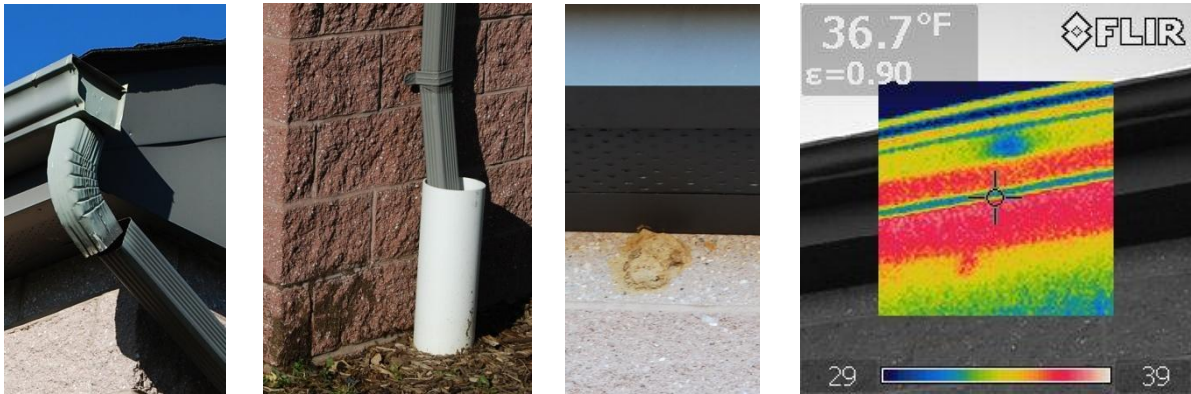
Dislocated downspouts and insect nesting with possible water or moisture damage detected
