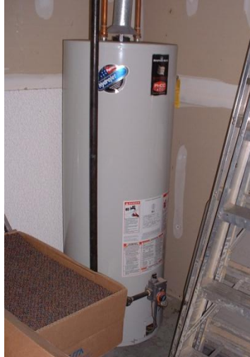
Domestic Hot Water heater
