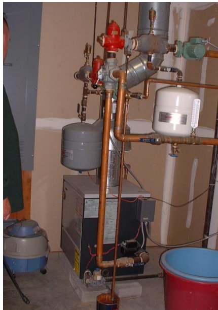
Slant / Fin Corp natural gas boiler
