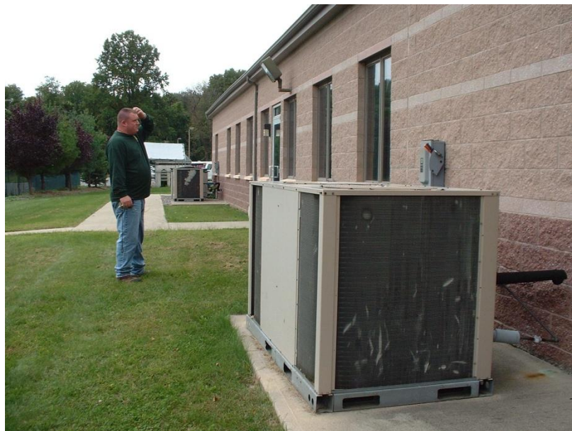
Two condensers for building DX cooling located outside the building
