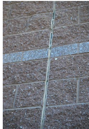
Cracked caulk in expansion joints
