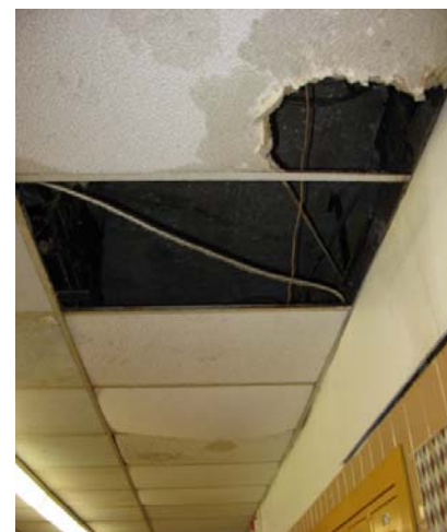
Water Damaged Drop Ceiling
