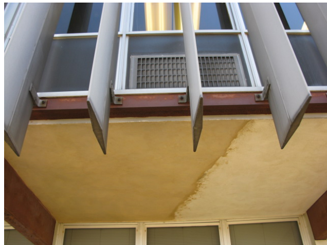
Water Damaged Exterior Soffit
