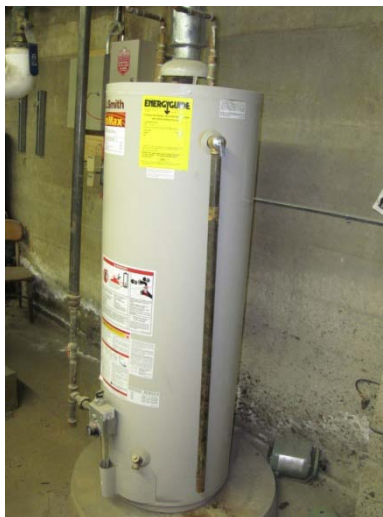
DHW tank in basement
