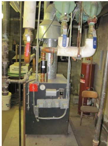
Natural gas-fired boiler in basement
