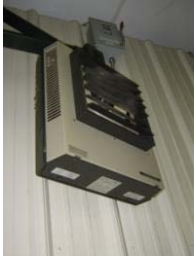
Electric unit heater
