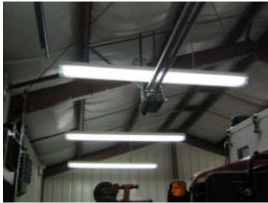
Interior Fluorescent Light Fixtures
