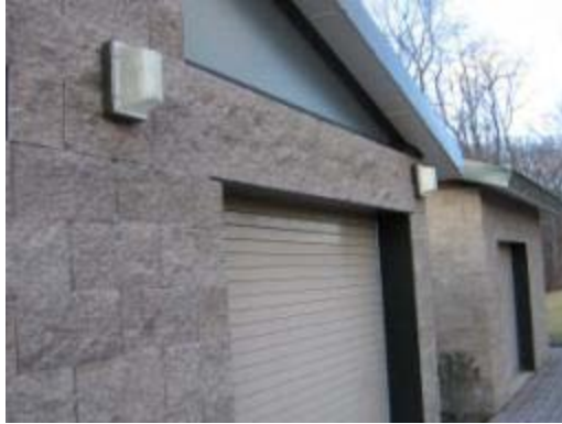
Photo – Exterior Metal Halide Fixtures
