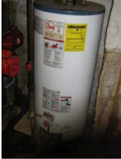
Domestic Hot Water heater
