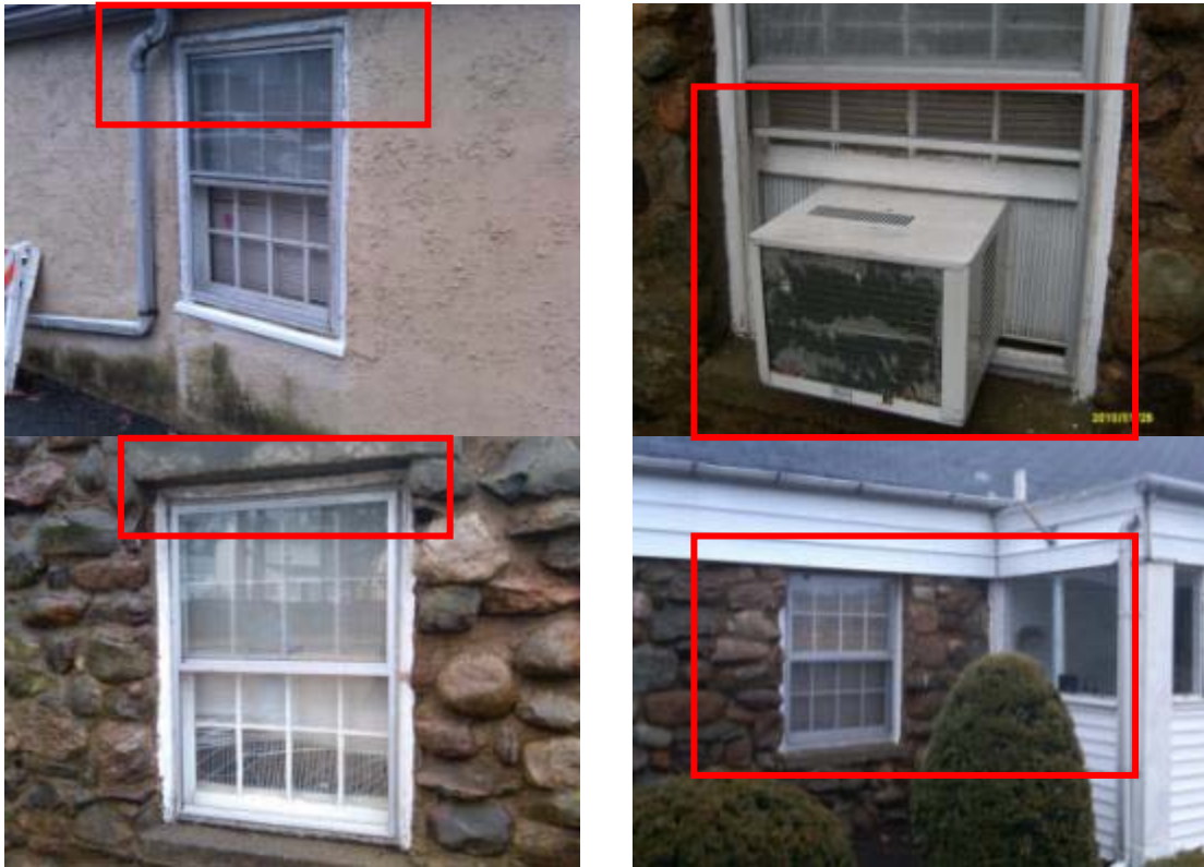
Damaged/ aged window frames, improperly sealed window A/C units, water pooling at window sill
