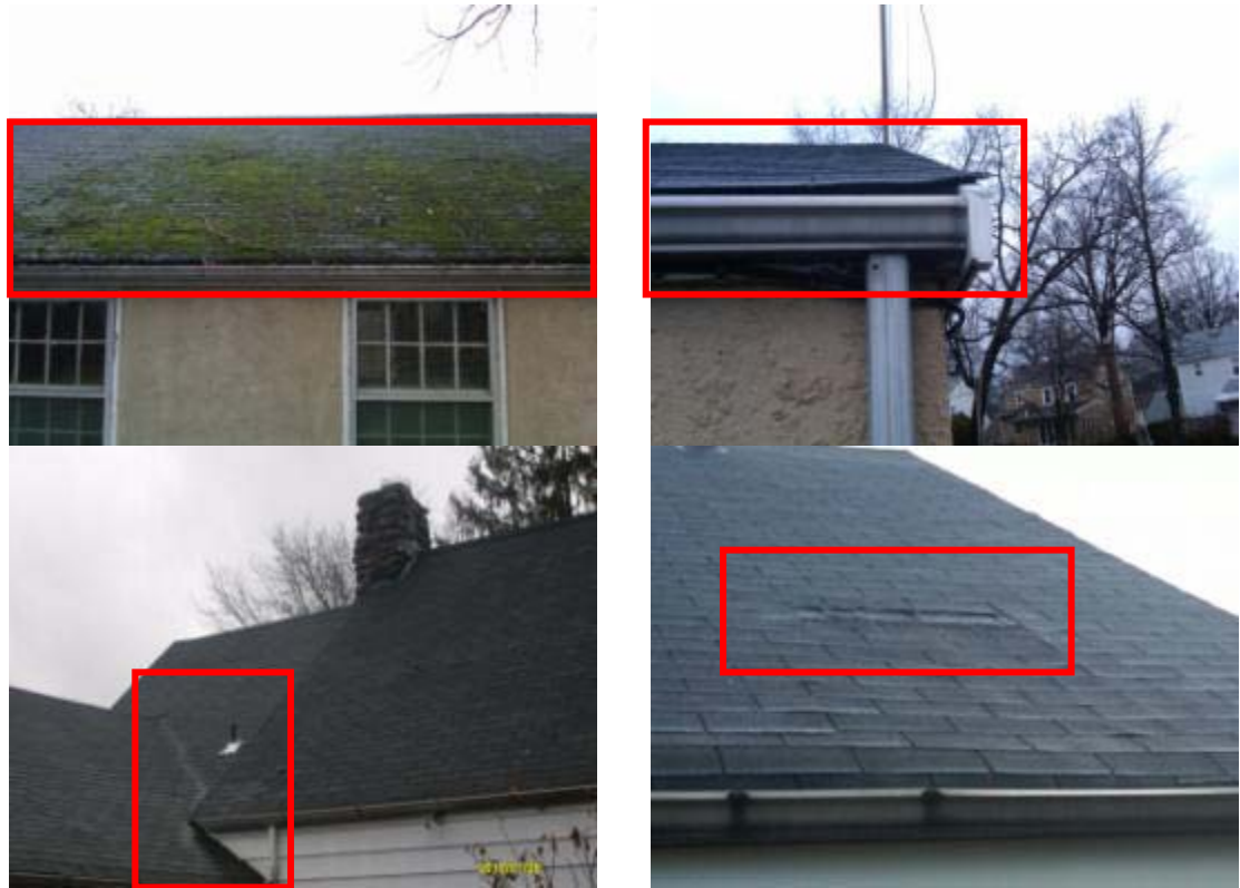
Typical asphalt shingle roof with mold, water damage and uncontrolled vegetation growth on the roof, missing and displaced shingles, defective gutters, and missing / ineffective flashing
