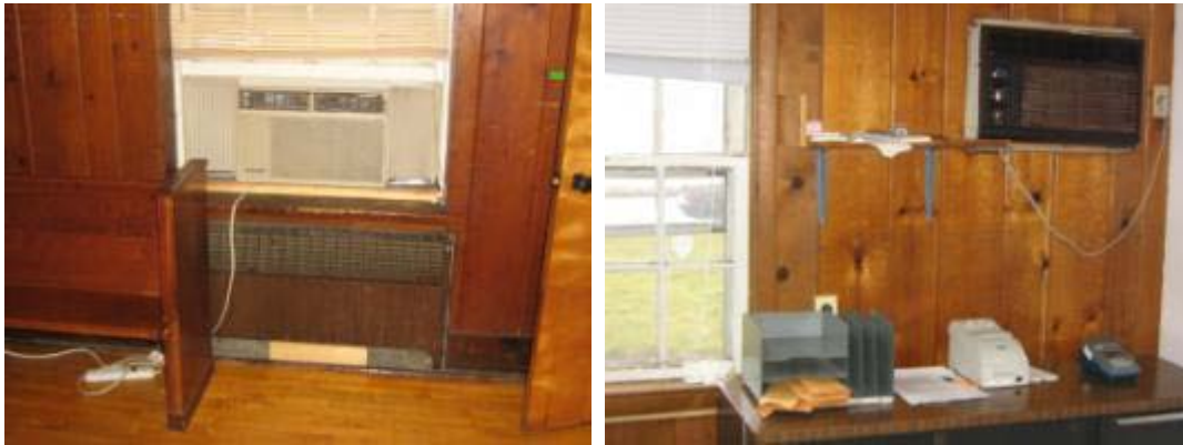
Thru-the-wall air conditioners
