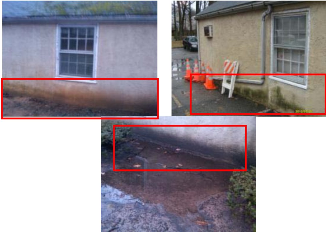
Water damage at base of the building and moisture seepage through cracks detected in the slab
