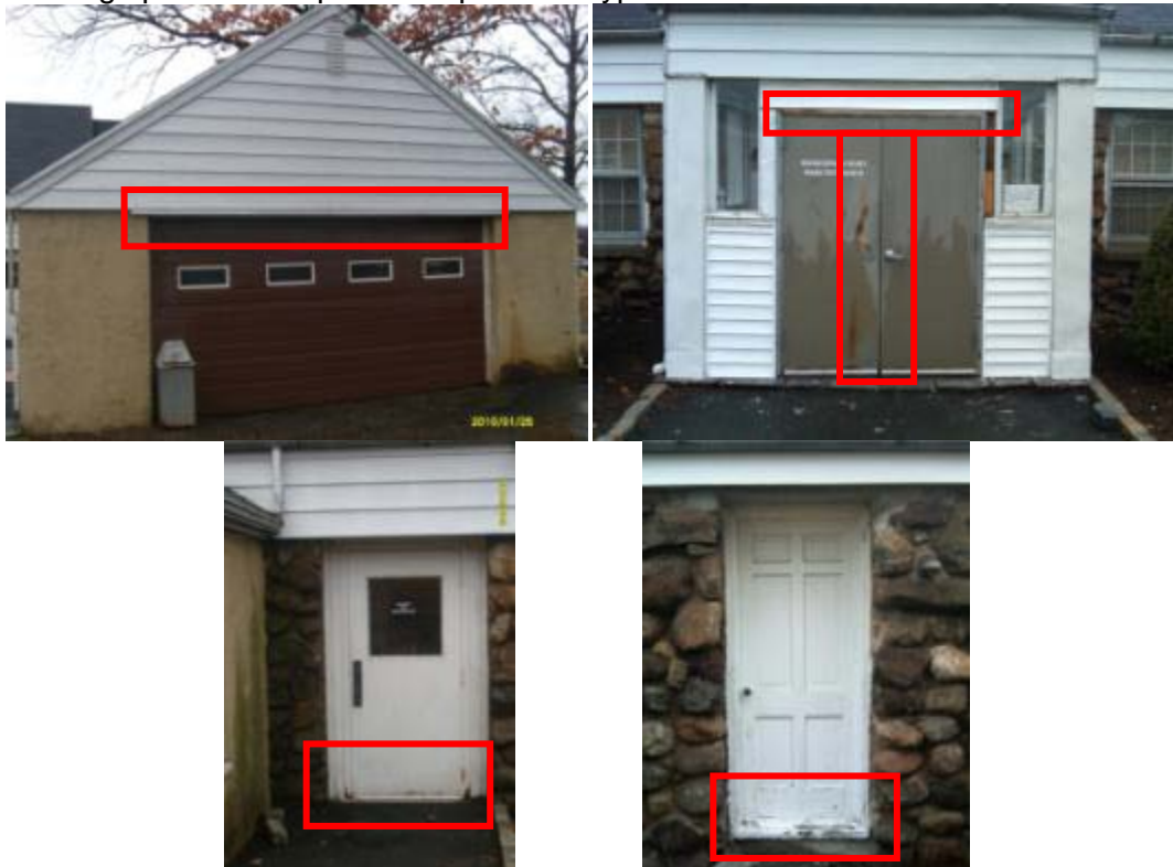
Damaged/ warped/ aged door frame
