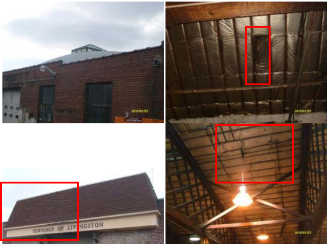
Examples of typical roof surfaces, missing asphalt shingles and damaged roof insulation.
