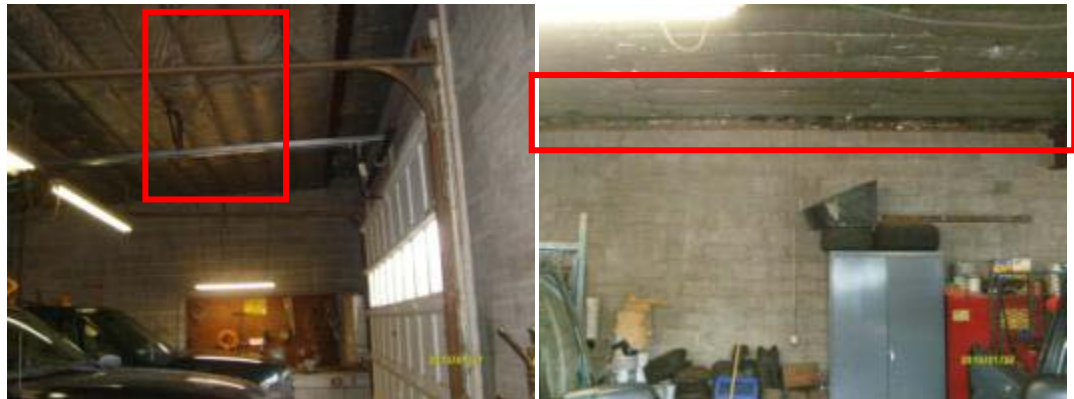
Sagging roof insulation showing signs of water damage
