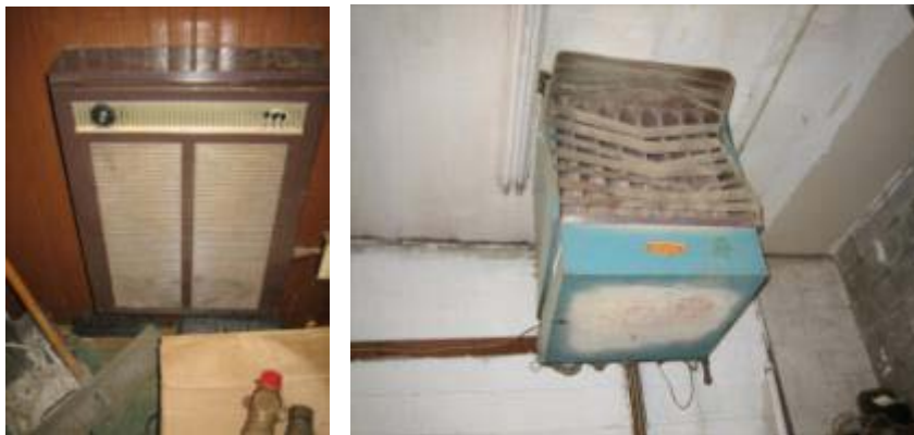
Electric unit heater in office, gas unit heater in rear garage
