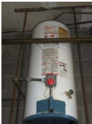
Domestic water heater
