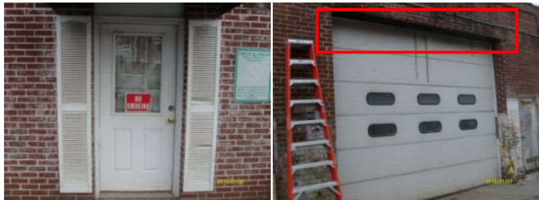
Typical door installations and some signs of water damaged overhead door frames
