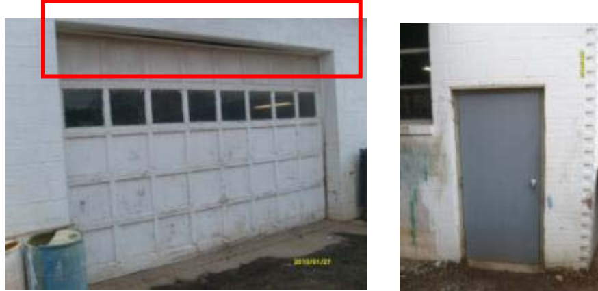
Typical door installations and some signs of exposed and damaged door frames
