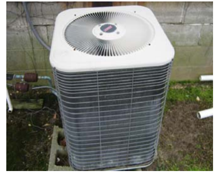
Condenser for the split AC system
