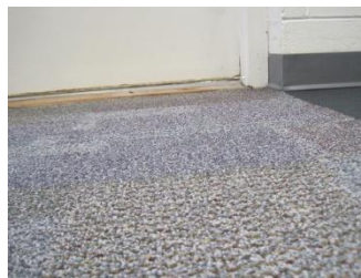
Missing/worn weather-stripping on meeting room exterior door
