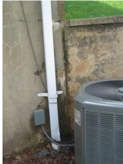
Mold/water damage on exterior finish
