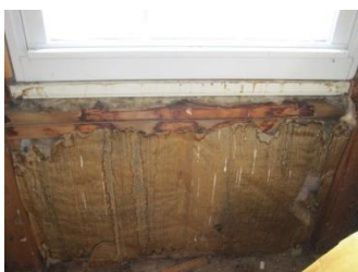
Signs of mold/water damage on interior finishes in attic
