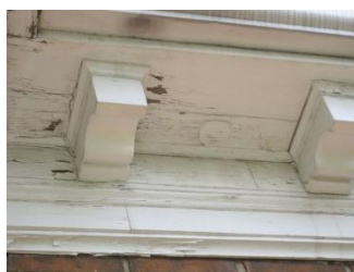
Soffit Vents along roof trim for attic air intake without air exhaust
