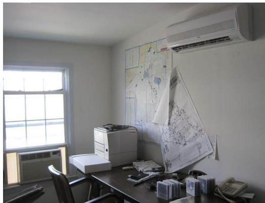
Server Room Wall Mounted Unit and AC Unit
