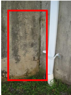
Mold/water damage on exterior finish
