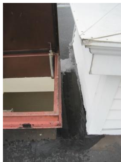
Signs of standing water/pooling near roof hatch
