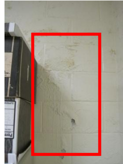
Mold/water damage on interior finish
