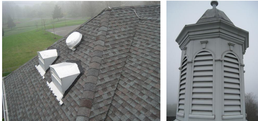
AHU-1 and AHU-2 Air Intakes and Fan (left); Cupola with Opening to Attic (right)
