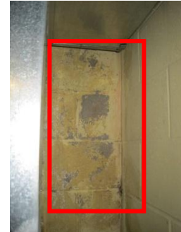
Mold/water damage on interior finish
