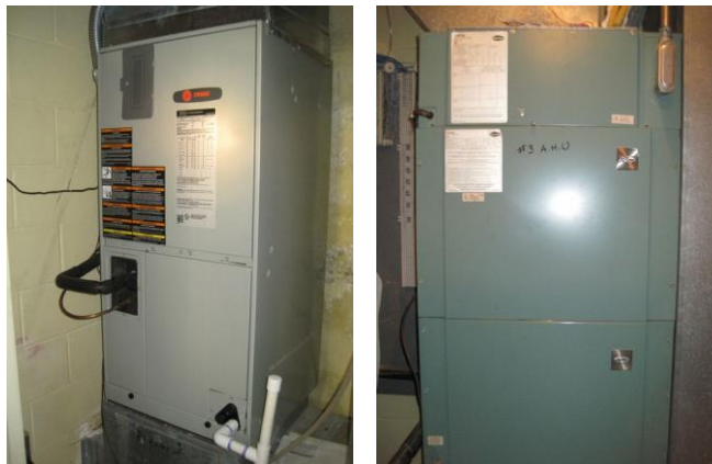
Heat Pumps, AHU-4 (left), AHU-3(right)
