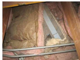
Uneven/ineffective attic insulation found in mechanical area of attic
