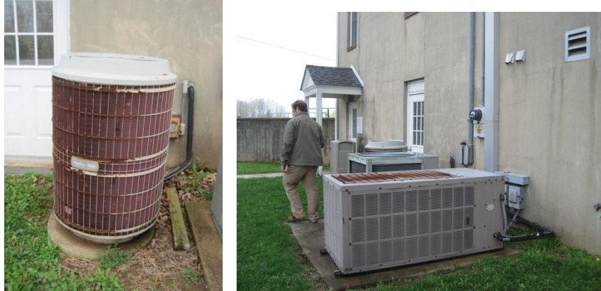
Outdoor Condensing Units for Heat Pumps, old and need replacement
