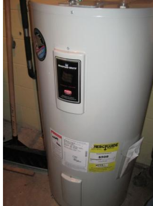
Domestic Hot Water Heater
