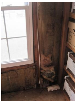
Signs of mold/water damage on interior finishes in attic
