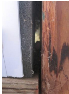
Gaps around window frames in attic
