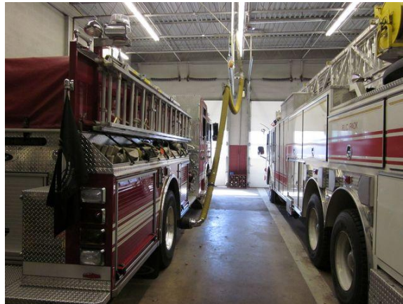
Ceiling mounted T8 fixtures in fire station
