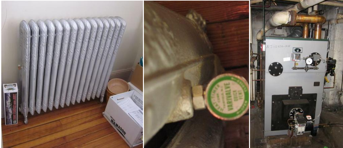
Treasurer office disconnected radiator, Vari-Valve, and Steam boiler
