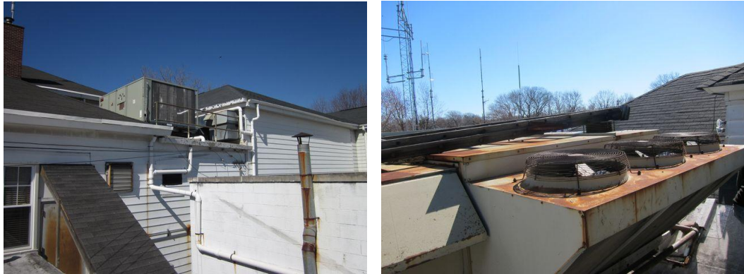
Library RTU (inaccessible) and Senior Center RTU (old and rusted)
