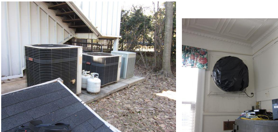
Condensing units on grade and a Fan covered with a plastic
