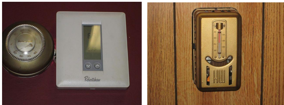
Fire department (manual and programmable thermostats) and Fire Marshall office manual thermostat
