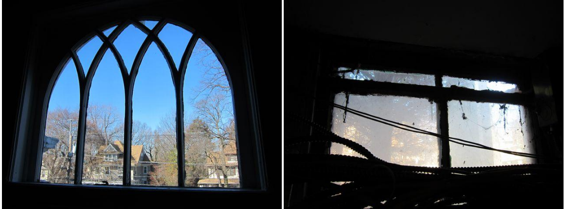
Single-glazed windows with ineffective wood frames – leading to cold drafts
