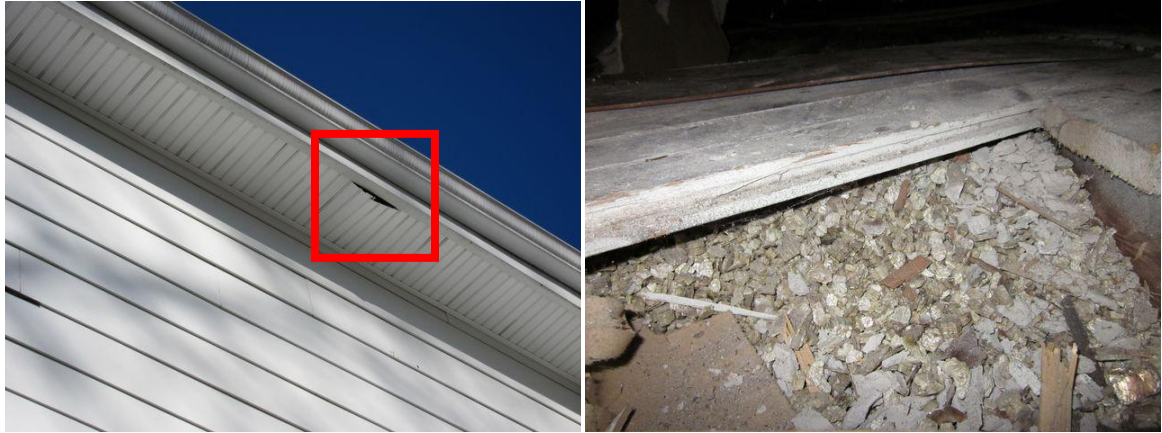
Deteriorating soffit and typical vermiculite attic insulation
