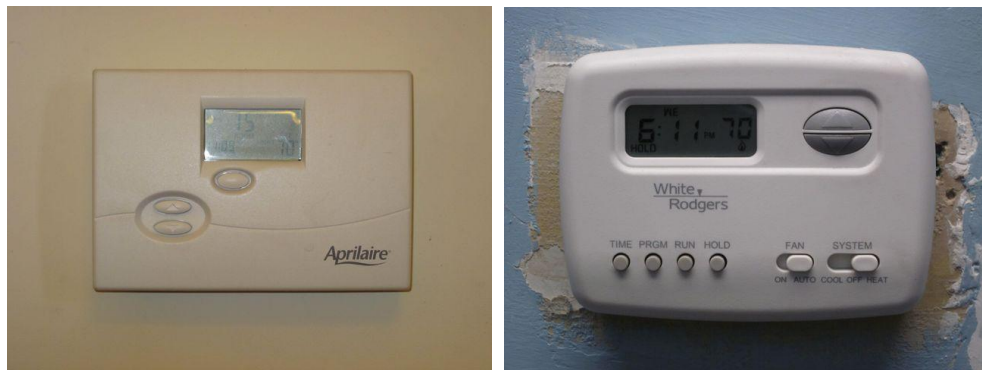
Health office and Police department – programmable thermostats
