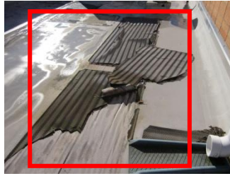
Delaminating roof membrane/patches due to slip guard tearing
