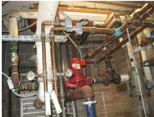
C Wing Hot Water Distribution Pump
