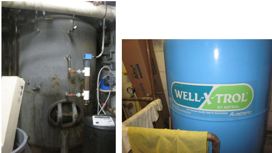
Main Cold Water Storage (left) and Annex Storage (right)
