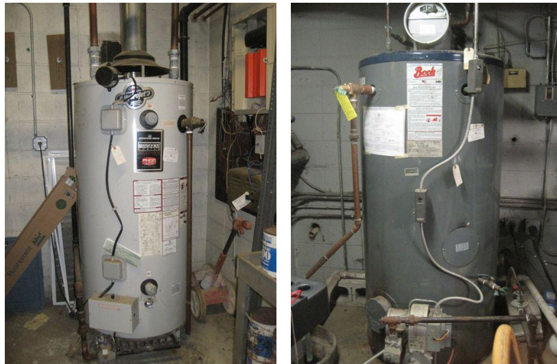
Two Natural Gas Heaters with Storage
