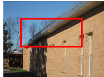
Sagging roof soffit
