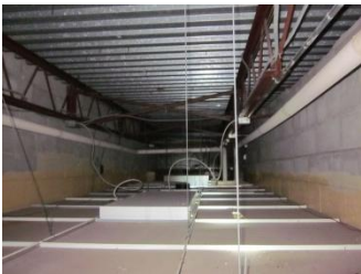
Missing ceiling insulation in D Wing
