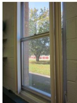
Single-glazed window with ineffective frame
