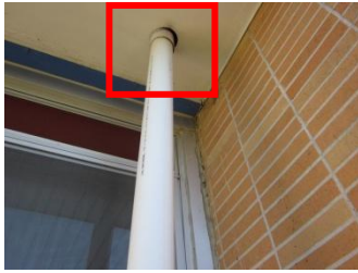
Un-caulked/un-sealed exterior wall penetrations
