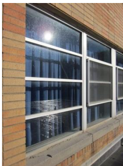
Single-glazed window with ineffective frame
