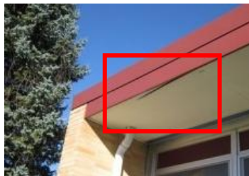
Damaged exterior trim
