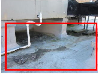
Signs of standing water/pooling
