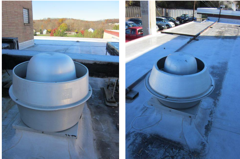
Typical Rooftop Exhaust Fans
