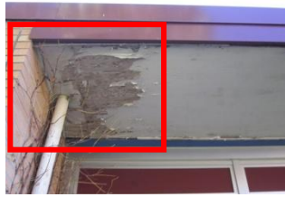
Deteriorating exterior wall finishes
