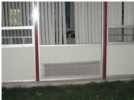
Outside Air intake for Unit Ventilators
