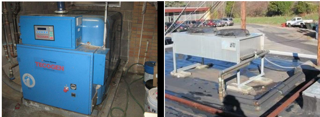
75.0 kW CoGeneration Unit; Air-Cooler on Roof for CoGen Coolant Water
