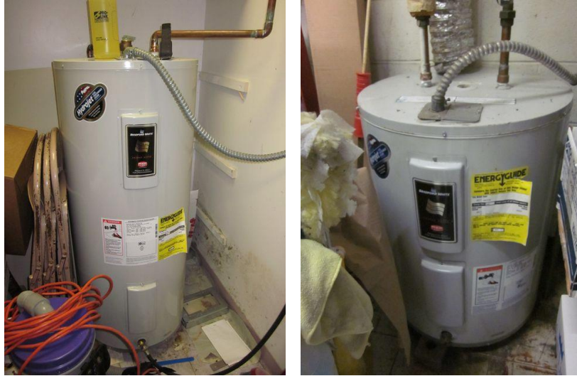
Electric Hot Water Heaters in Janitor Closets
