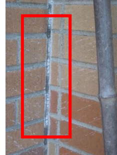
Cracked/deteriorated mortar joints
