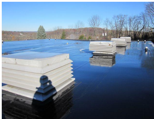
Exhaust Dampers on Gym Roof
