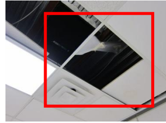
Leak in Room 35 from roof
