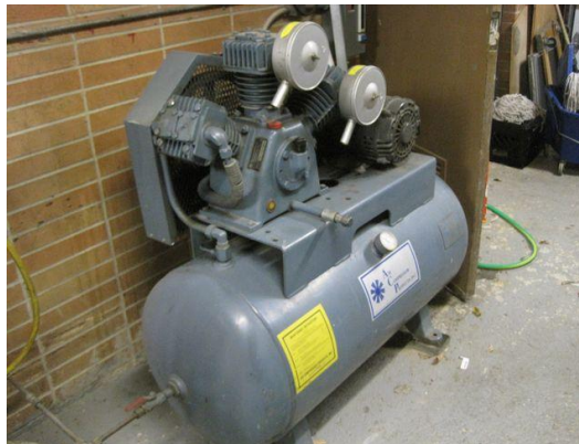
Air Compressor for Pneumatic Valves
