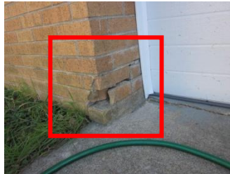
Cracked/deteriorated bricks and mortar joints
