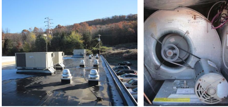
Four Gas-Fired Rooftop Units; RTU supply fan and motor
