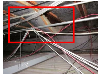
Sagging attic insulation found
