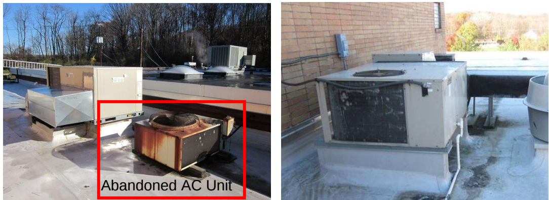
Main Office RTU Cooling Only and Abandoned Unit; Teachers Lounge RTU Cooling Only
