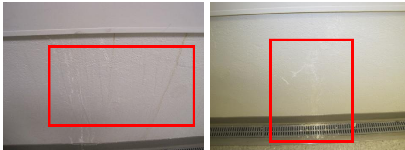
Some structural hairline cracks detected in the foundation wall and moisture on walls popping out the wall finish in the basement
