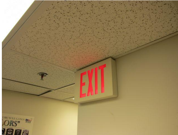
Typical LED Exit Signs
