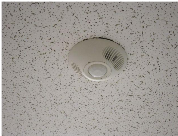
Typical bathroom occupancy sensor
