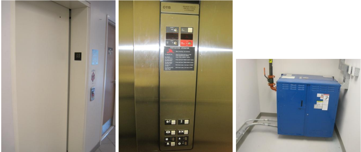
Otis elevator (above), outside (left) and inside (center) and hydraulic system (right)
