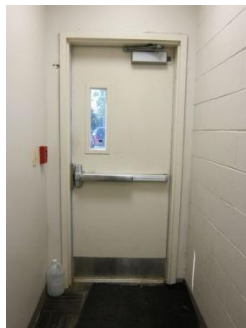
Damaged/warped door frame
