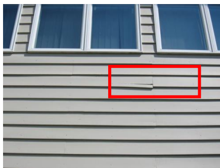
Damaged exterior wall finishes
