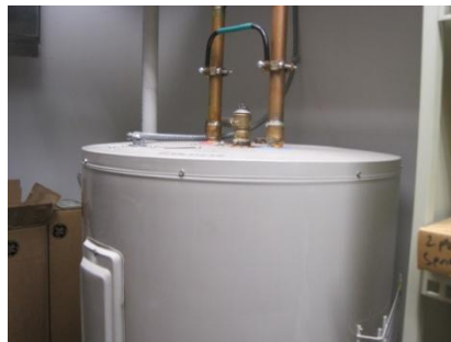
Borough Hall electric DHW heater - distribution piping should be insulated
