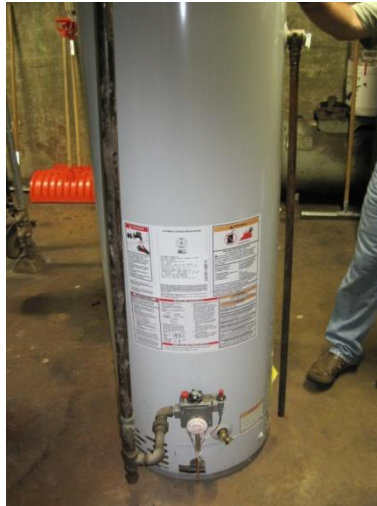
Gas fired 50 gal DHW heater serving the Fire Department building (left)
