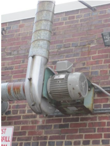
Wall mounted truck exhaust fan (left)
