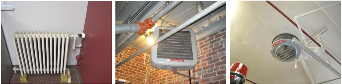
Steam radiator & manual adjustment
