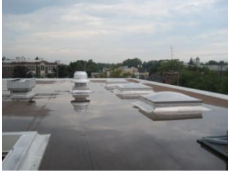
Standing water due to insufficient roof pitch
