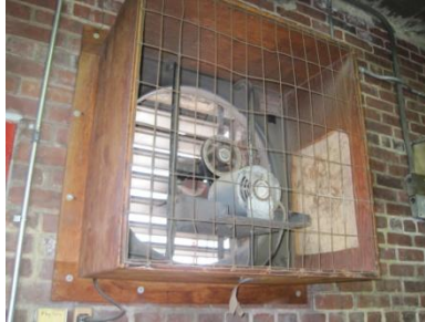
Kitchen exhaust fan (right)
