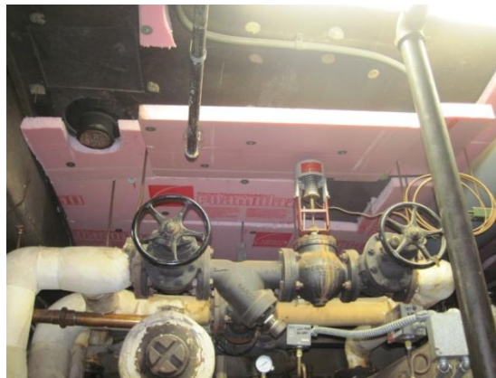
Attempt to sound-proof Boiler room from Communications room above
