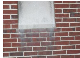
Efflorescence on brick façade below window due to missing flashing
