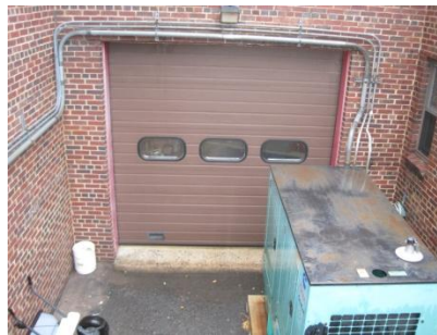
Onan GenSet emergency generator
