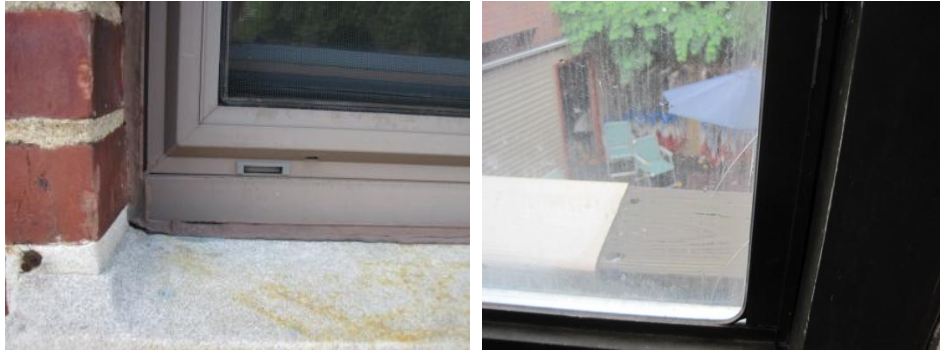
Broken sealants in windows and aged caulk around window perimeter
