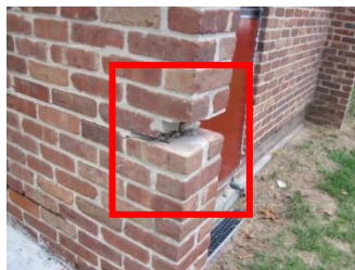
Damaged exterior brick
