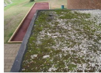
Uncontrolled vegetation growth on roof
