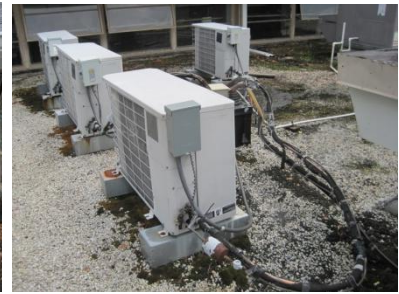
Four ductless mini split air conditioners
