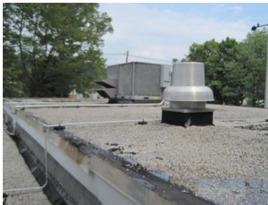
Benson meeting room exhaust fan;
