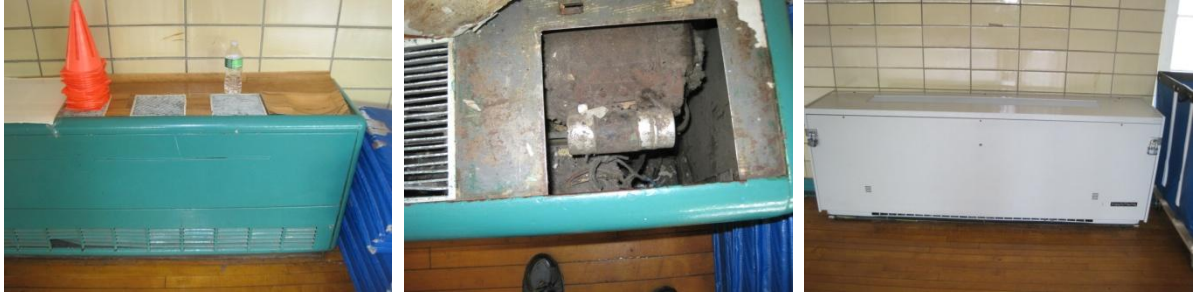
Gym Nesbitt unit ventilators, 1955 vintage (left and center) and 2009 newer unit (right) - Not the best application where there is a high tendency for units to be banged by balls
