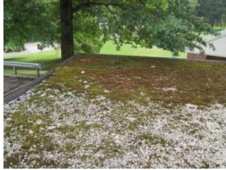
Uncontrolled vegetation growth on roof
