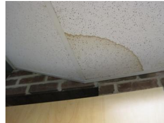
Signs of water damage on ceiling tile
