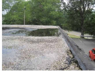
Standing water on roof
