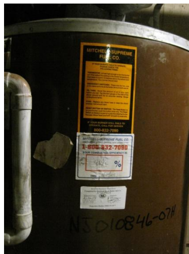
Fuel oil fired 86 gal DHW heater serving the Community Center building (left)
