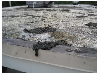
Uncontrolled moss muck on roof
