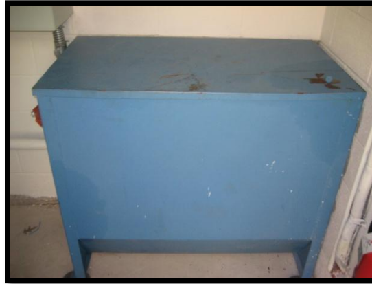
Hydraulic elevator motor
