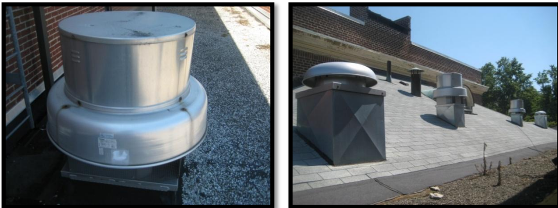
Typical rooftop exhaust fan units
