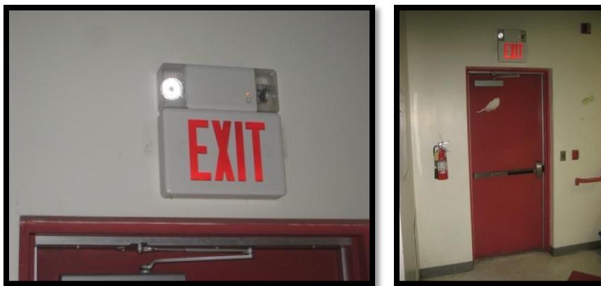
Typical LED exit lighting
