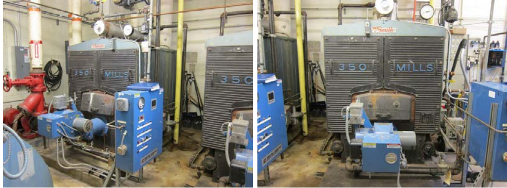
Two H.B. Smith 350 Mills boilers
