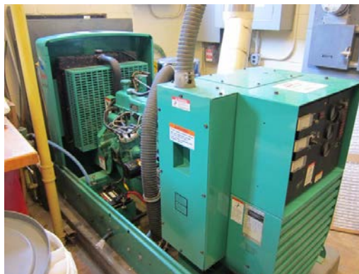
35 kW natural gas generator
