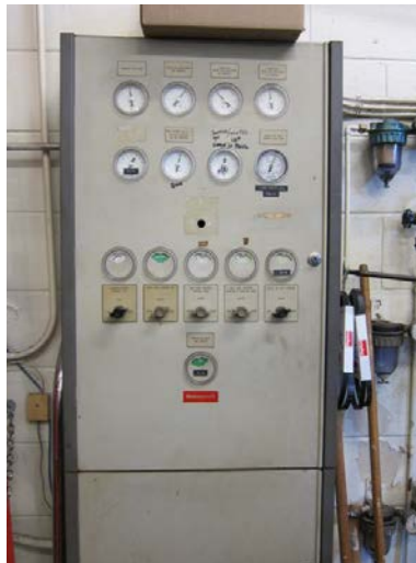
Honeywell control panel
