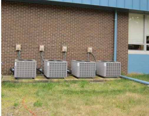
Condensing units connected to four units
