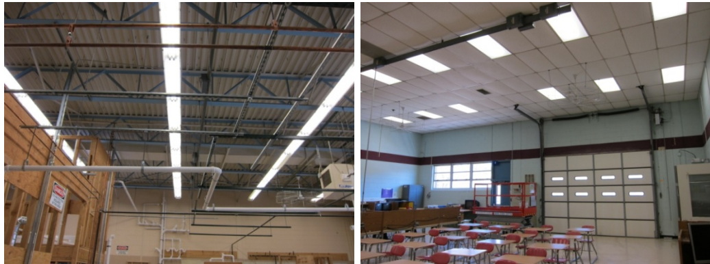
Typical interior T8 lighting (L); and typical T8 lighting in shop/classrooms (R)
