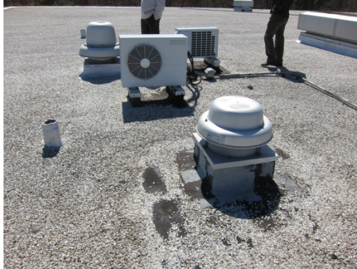
Deteriorating EPDM and lack of gravel BUR
