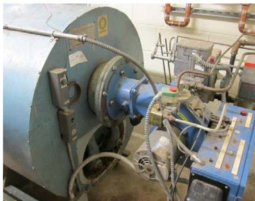
Patterson Kelley Domestic Hot Water Heater
