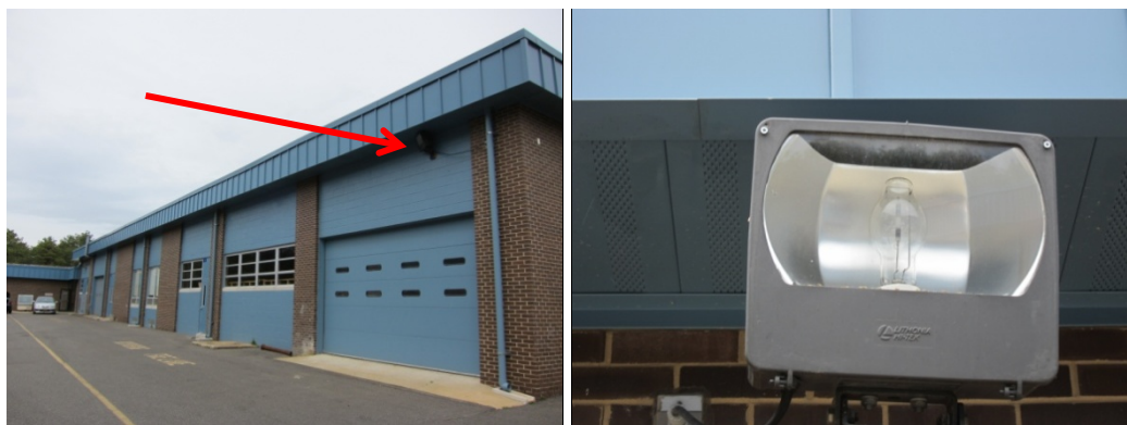
Typical high pressure sodium wall pack fixtures.
